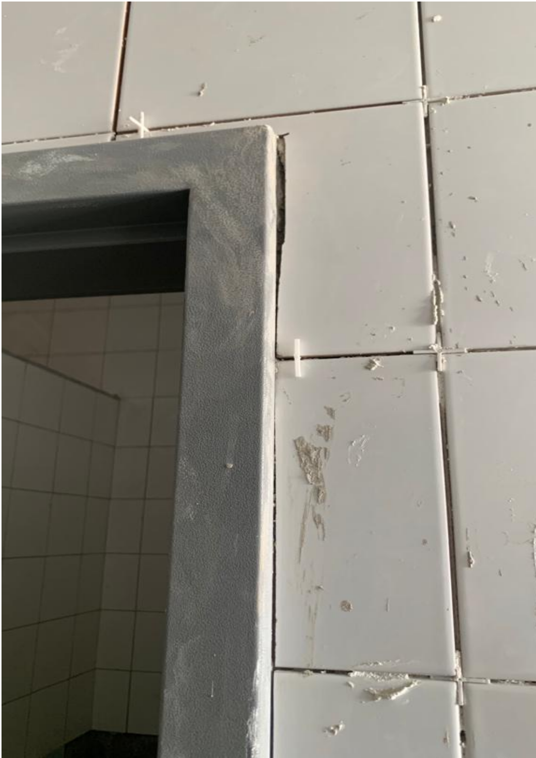
Unacceptable finishing of ceramic tiles at the door frames
