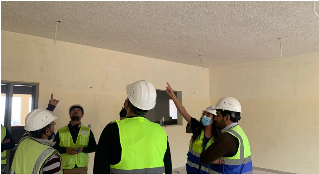
Defects in accoustical plastering
