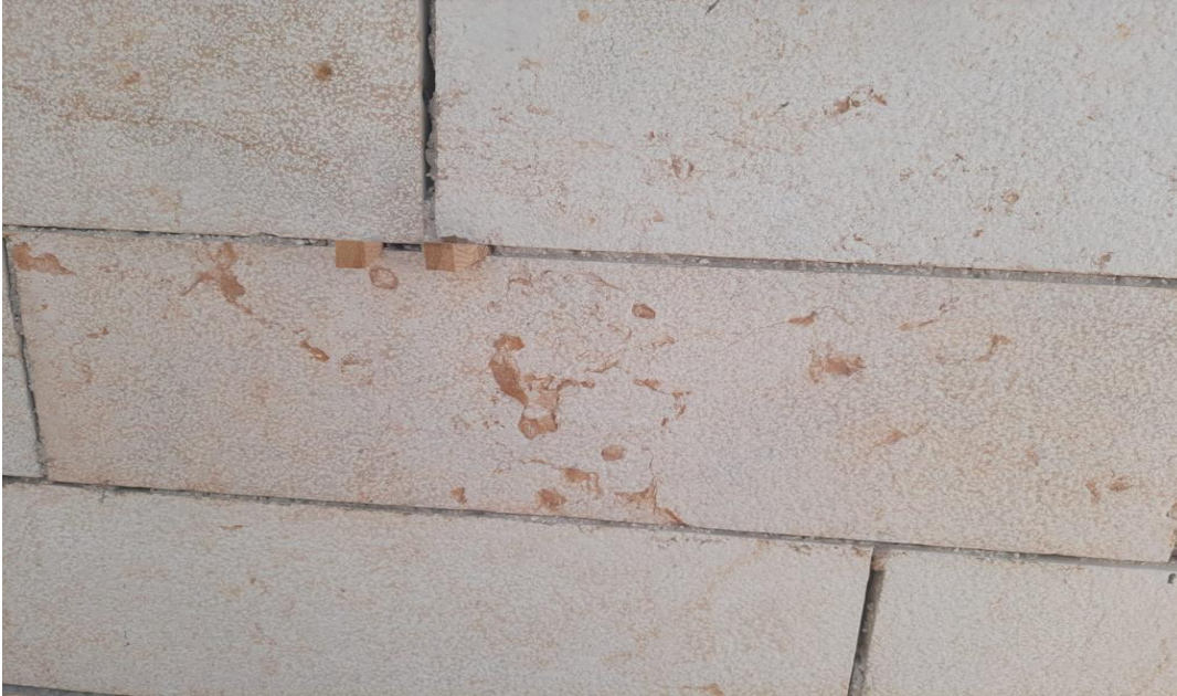
Defected built stones
