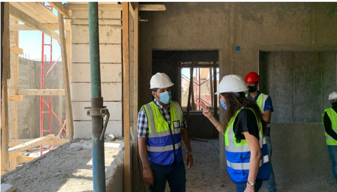
Discussing connection between backing concrete behind stone and window jamb with the internal finishing
