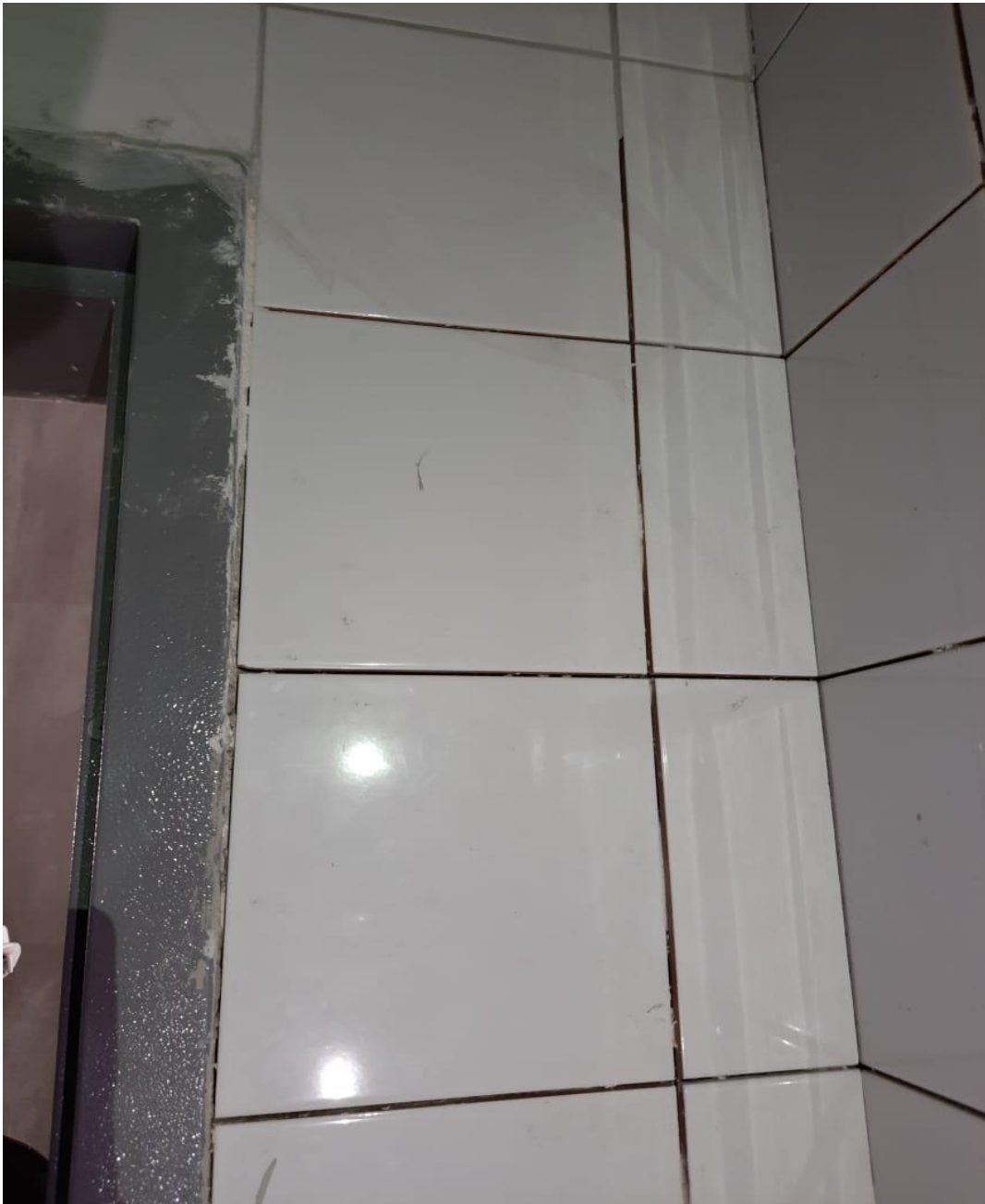
Inappropriate finishing of tiles at the door frames
