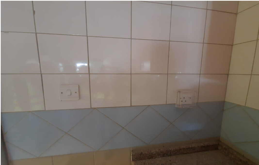
Inappropriate electrical sockets location at the internal façade
