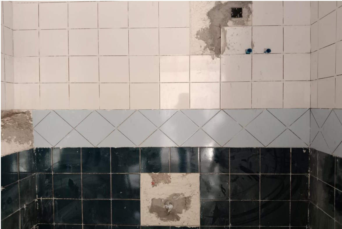
Defected tiling at toilets (2)
