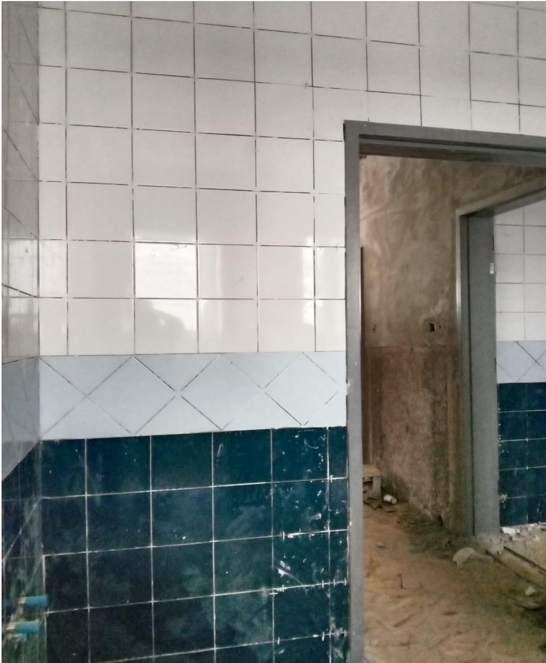
Defected tiling at toilets (1)
