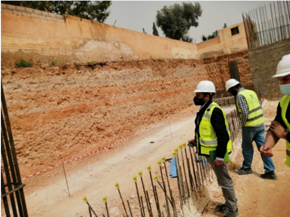
Reviewing the encroaching neighbor's wall
