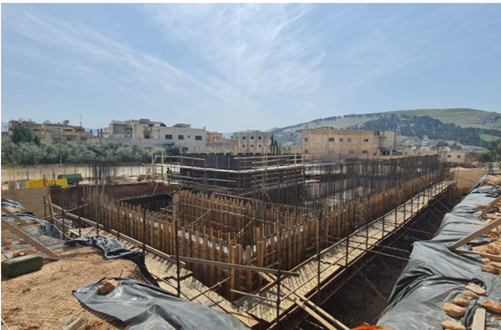
General view of basement floor and fair-face formwork for underground water tank- (30/03/2021)
