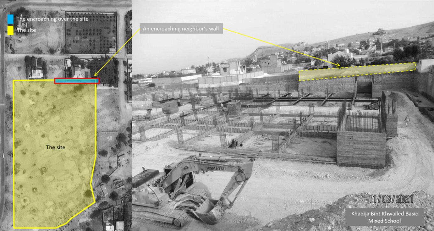
Figure 1. An encroaching neighbor's wall
