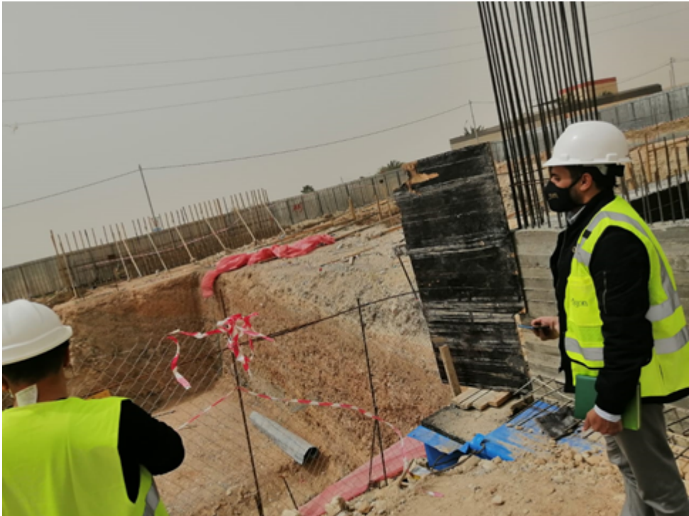
The location of underground water tank is surrounded by safety fence
