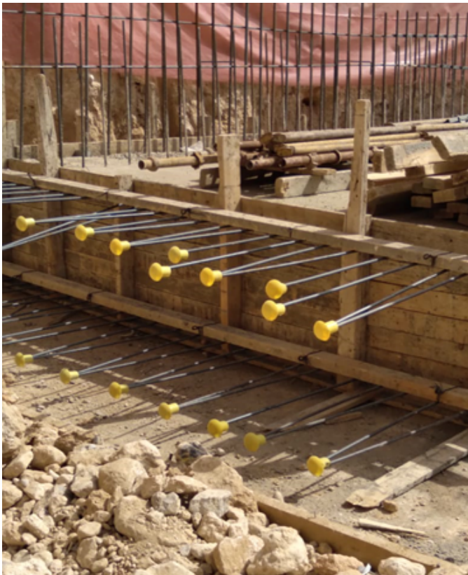
Safety measures on the construction site using safety caps on steel rods
