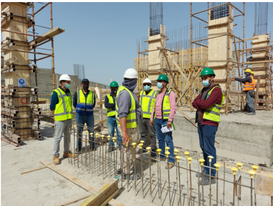
Safety measures on the construction site using safety caps on steel rods
