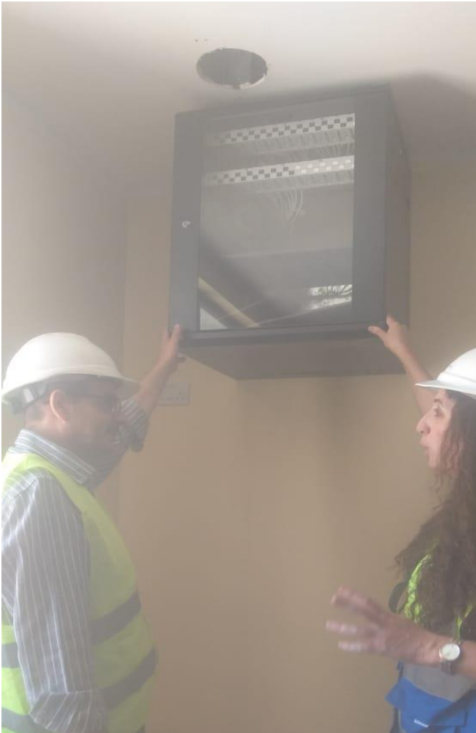
Damage in patch panel cabinet
