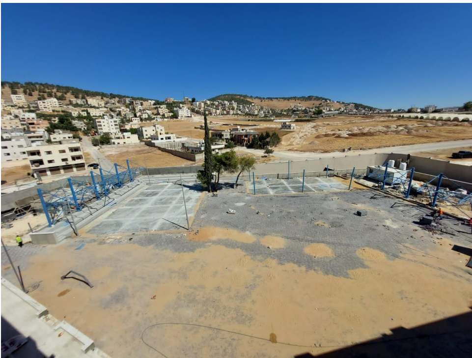
External works (shadings and interlock) for the playground and morning assembly area
