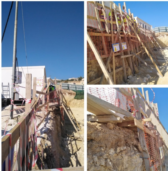
Figure #2: The Contractor office trailers were fixed on the top edge of an excavation area close to the site entrance – Potential Risk of Collapse. Photo credit: Odai Tawalbeh, 11/18/2020
