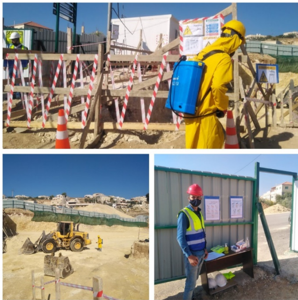
Figure #4: The temporary gate properly secured and guarded; High visibility clothing; All incoming and outgoing vehicles were disinfected by spraying materials; Warning tapes and warning signs available; and Work sites and facilities were cleaned on a daily basis using sterile materials. Photo credit: Odai Tawalbeh, 11/18/2020
