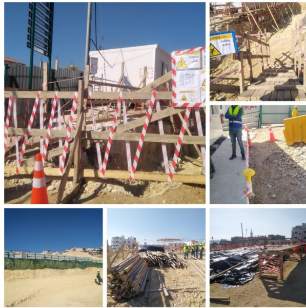
Figure #3: Sides of excavation were supported by temporary railing system; Safety mushroom caps were fixed to all R/F bars; and Proper material storage on site. Photo credit: Odai Tawalbeh. 11/18/2020
