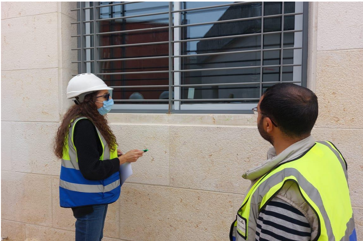
Defects in the steel protection screen
