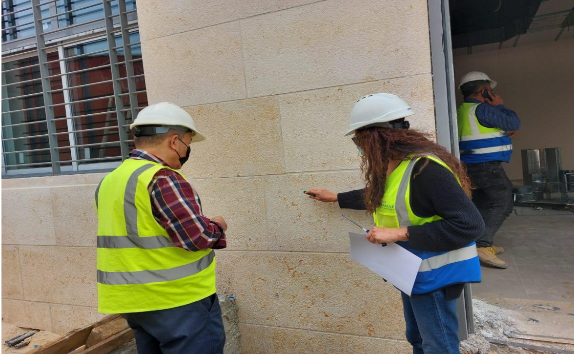
Not removed defected stones
