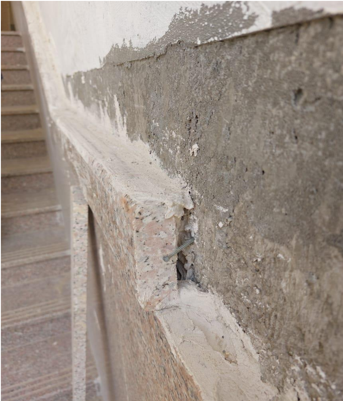
Defects in installing the granite coping
