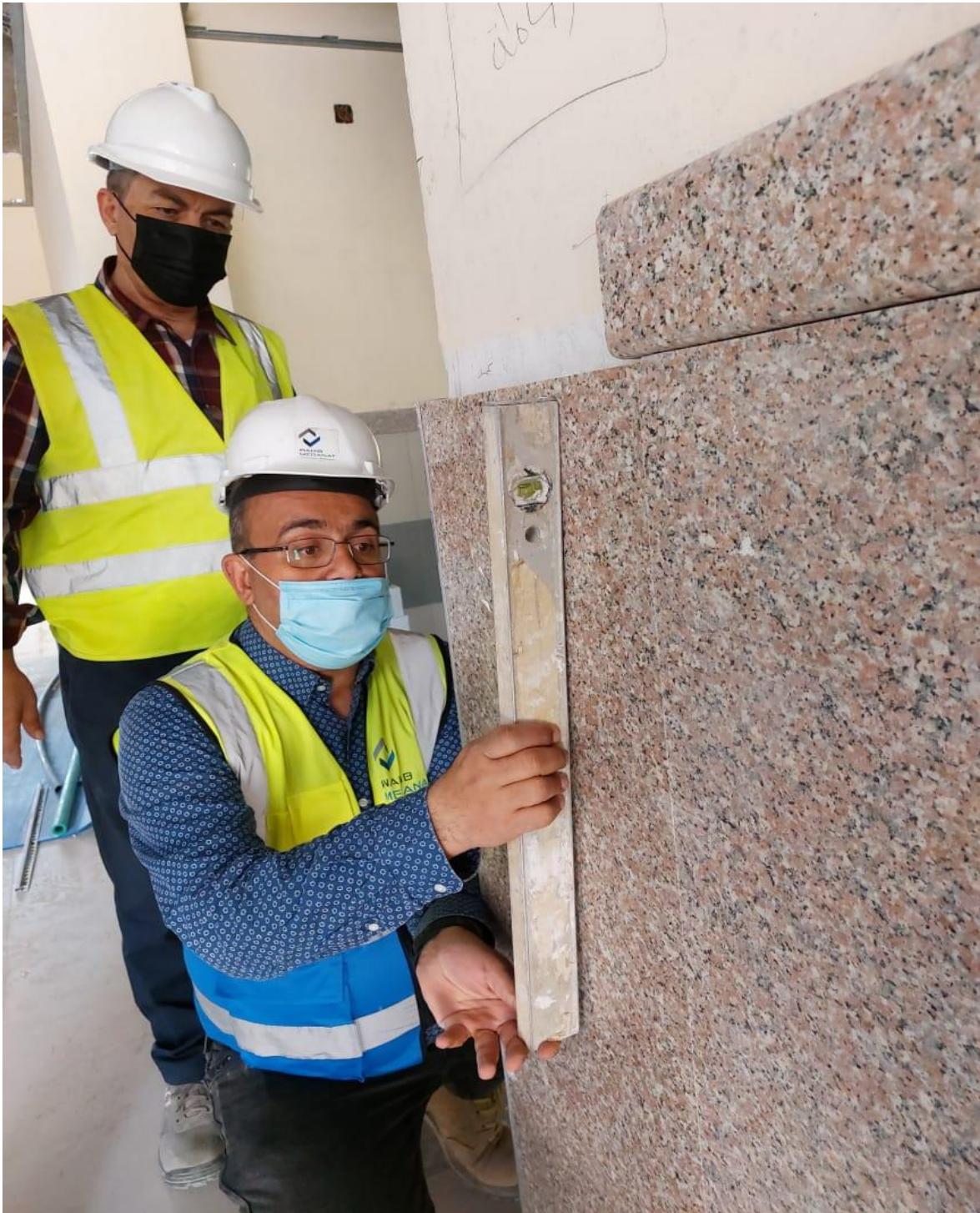
Defects in installing the granite cladding
