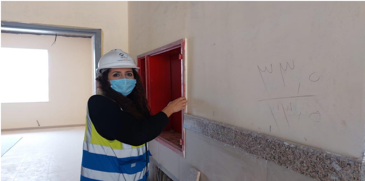
Unacceptable filling around the cabinets
