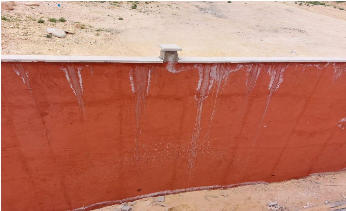
White color appears on the external plastering
