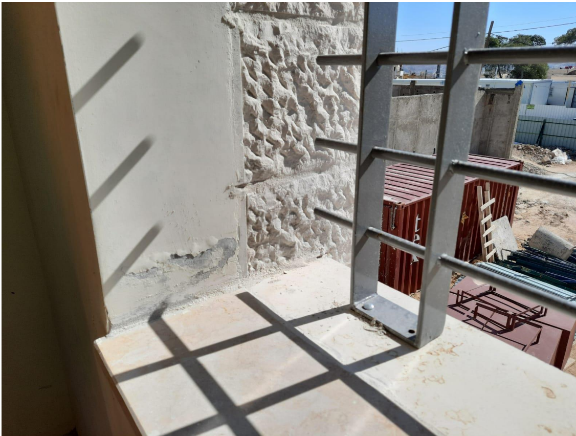
Defects in the window jambs
