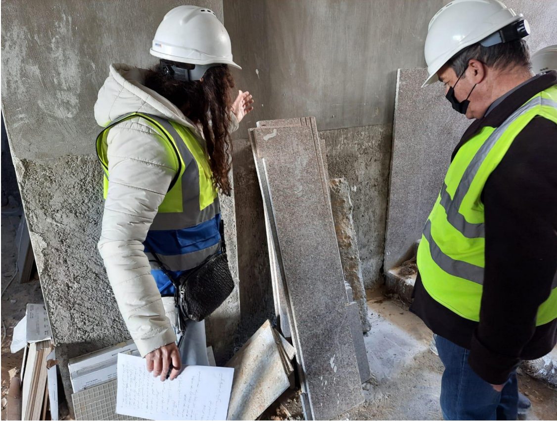
Inspecting the newly delivered granite pieces for staircase walls. The team observed that the newly delivered quantities have the same defect
