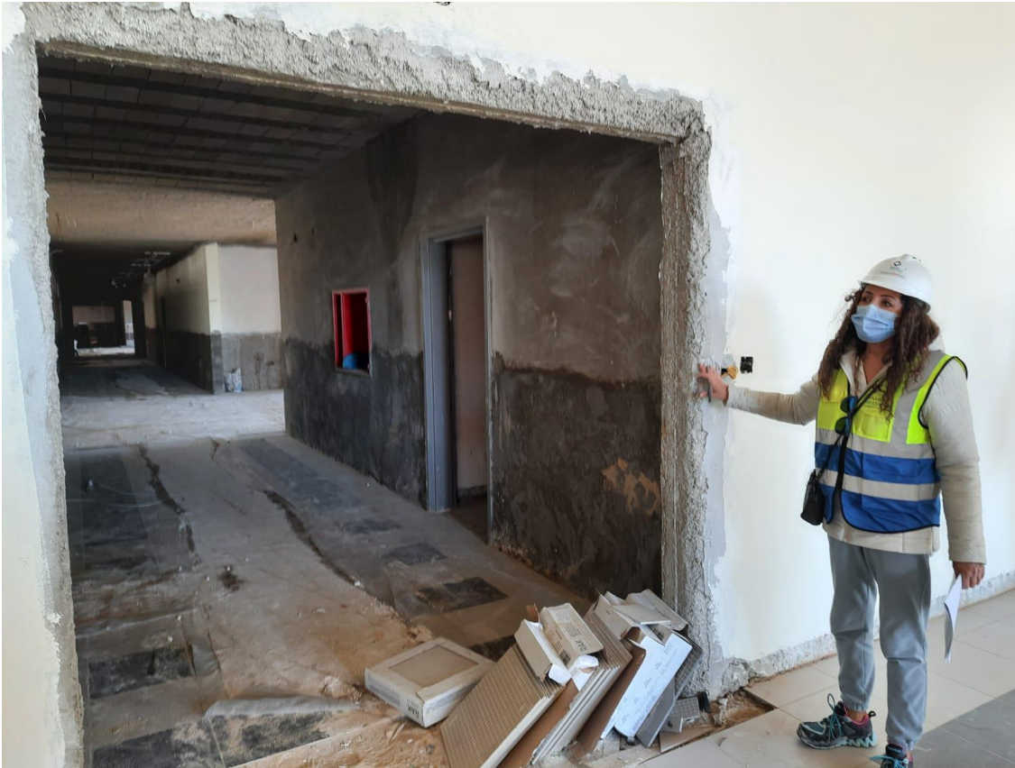
Fire rated door frame not installed
