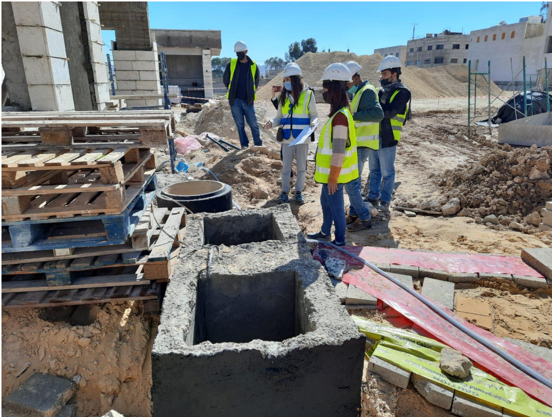
Inspecting the wrong execution of electromechanical manholes
