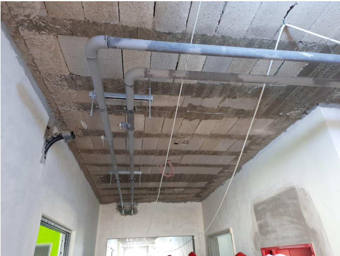
Executed heating pipes network
