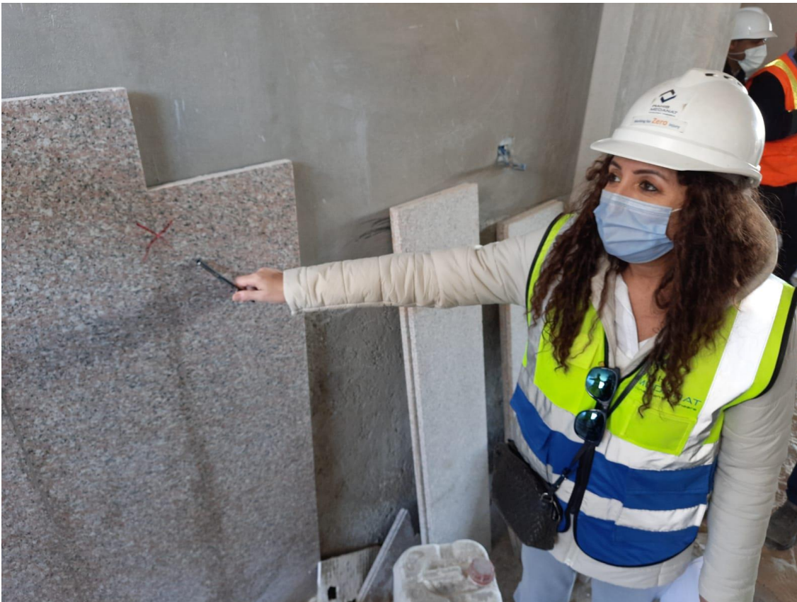
Inspecting the defects in tiling of granite for staircase walls
