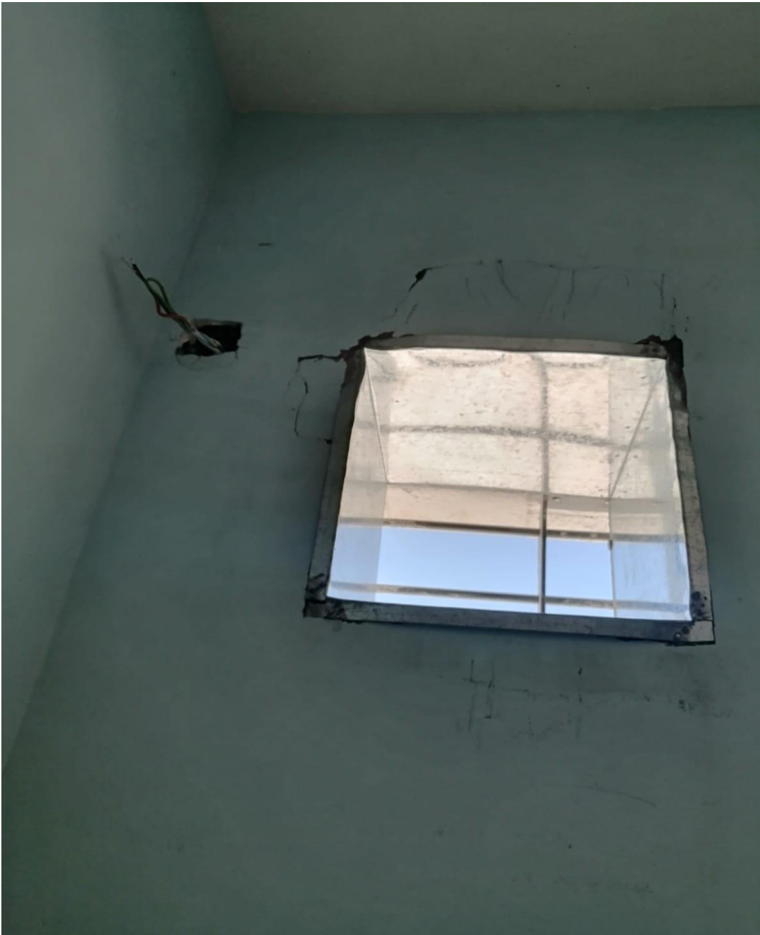
Damaged base plate and damaged wall around the wall fans
