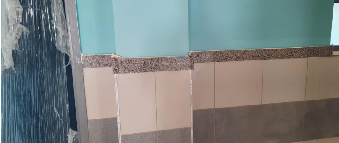
Rectifying the waving in plastering and painting of walls at the corridors
