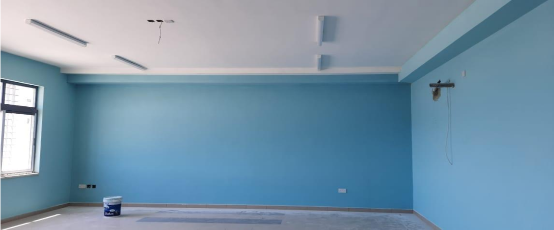
Incorrect installation of the gypsum board
