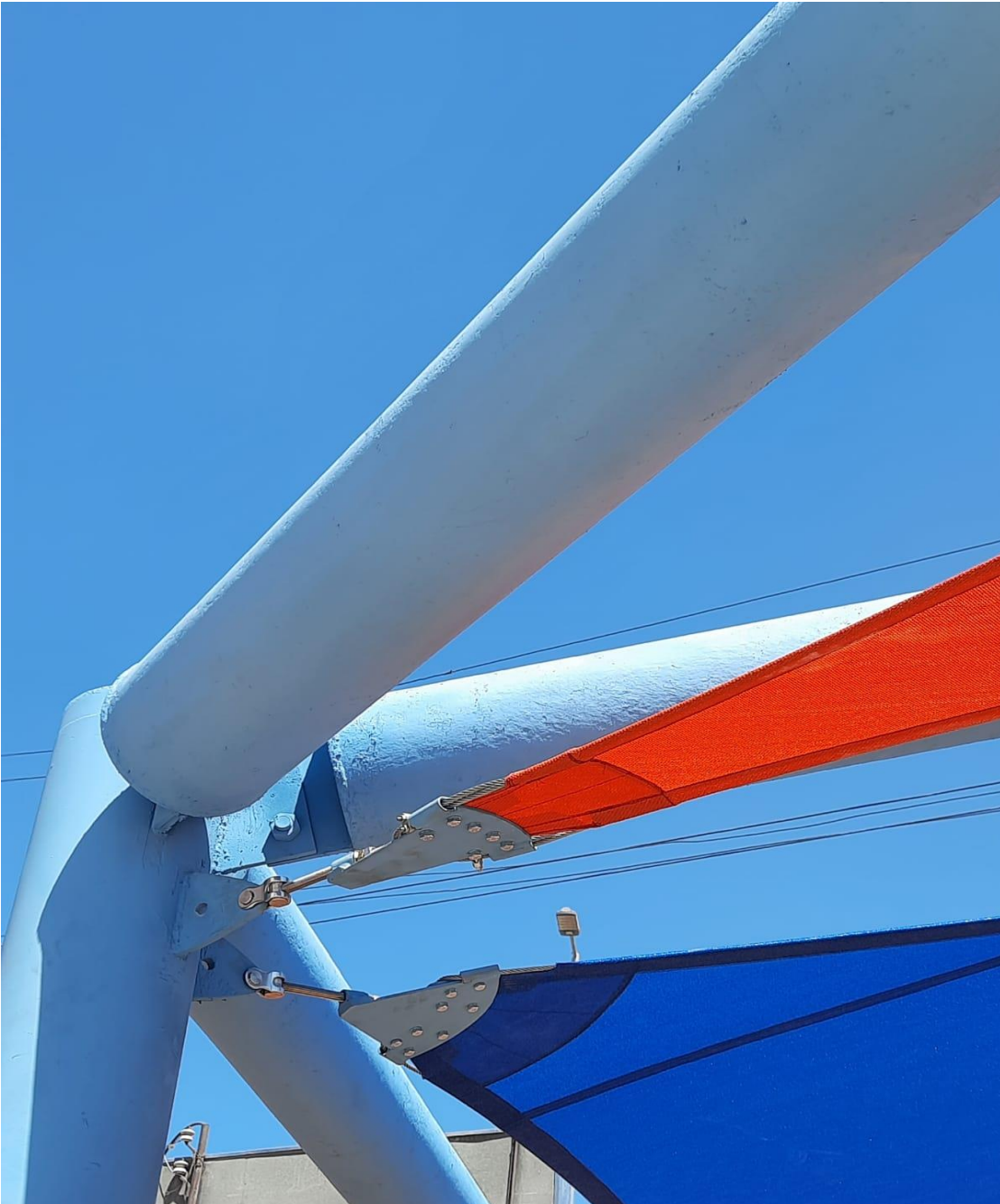
Defects in the painting of the horizontal pipes of the shading. Untight fabric
