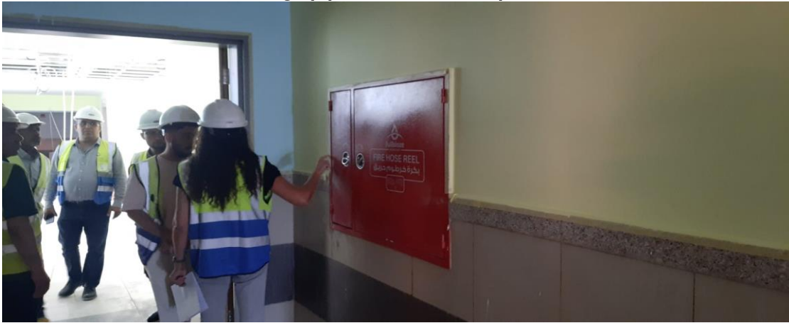
Finishing around fire hose cabinets is not finished as agreed upon previously
