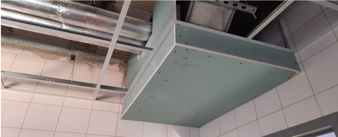
Suspended ceiling at the women toilet has wrong level
