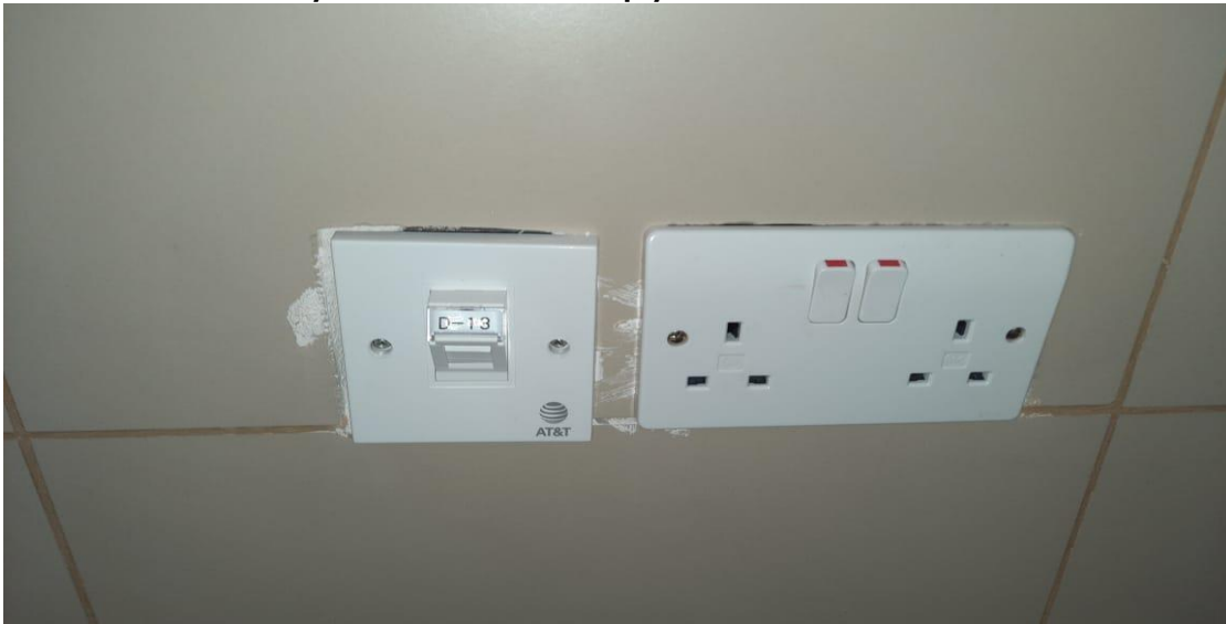
Defects in the finishing around the electrical sockets
