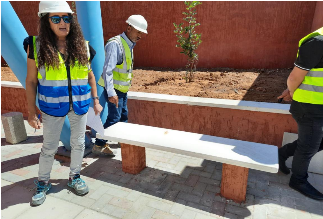
External benches supports not colored and the stone is one piece not two
