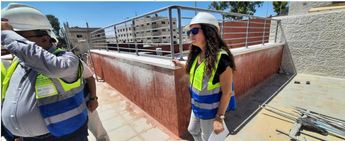
Dirt at the colored plastering
