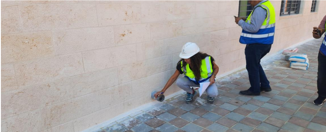
Protrusion of rainwater drainage pipe is more than required
