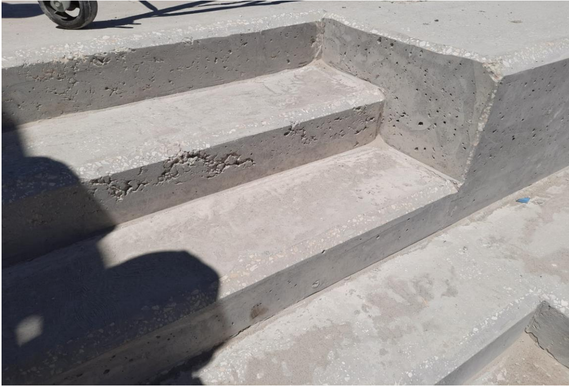
Voids in the casted concrete of the amphitheater
