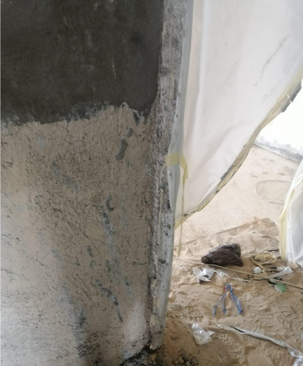
Removal of door frame with wrong dimension
