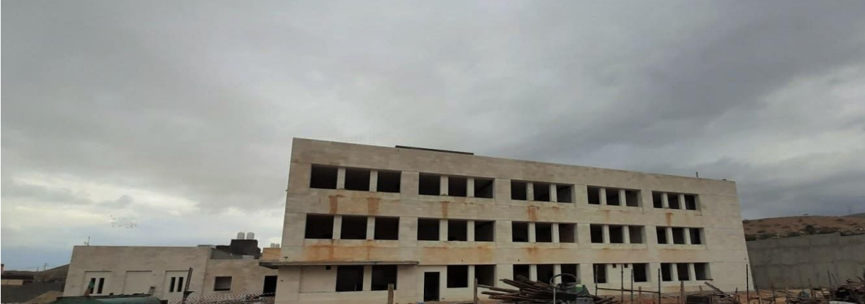
Dirts on the built stones
