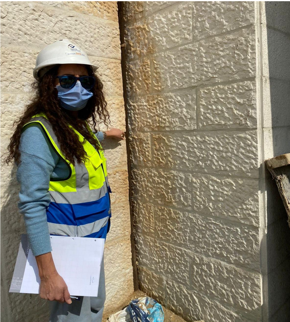
Dirts on the built stones
