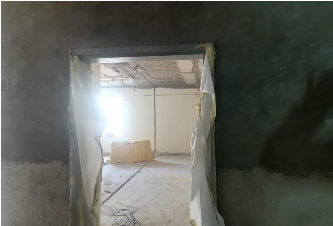
Door frame with wrong dimensions
