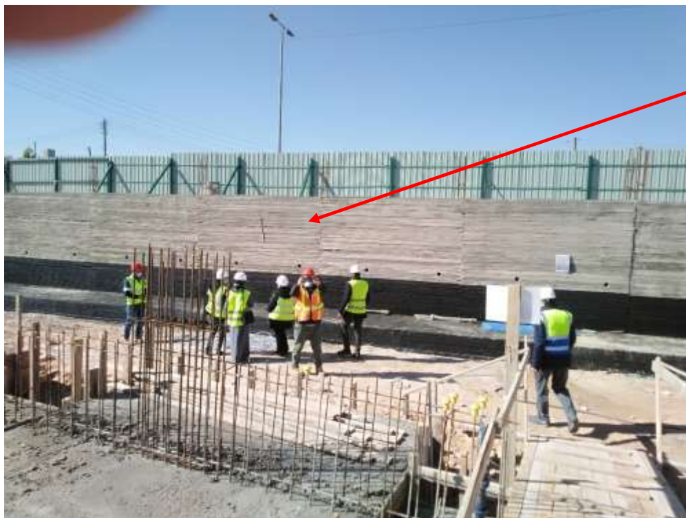
FIGURE #05: The construction of boundary walls nearby to Road is ongoing Photo credit: Osama Obeid January 24 2021
