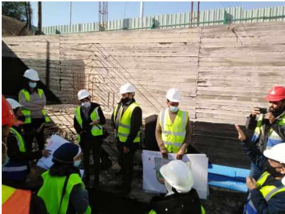
FIGURE #03 : During the site tour to inspect the construction works (Boundary walls and foundations) Photo credit: Osama Obeid January 24, 2021
