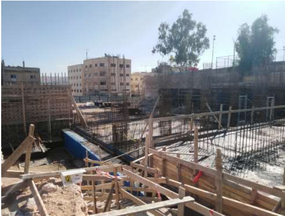
FIGURE #0& 09: New construction building will consist four floors and roof (basement, ground floor, first floor and second floor). The total area is 5700 sq.m and external area is 5600 sq.m including Basketball Court works Construction of building's foundation is completed
