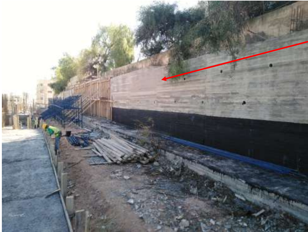
FIGURE #04: The construction of boundary walls adjacent to neighbor is ongoing Photo credit: Osama Obeid January 24 2021
