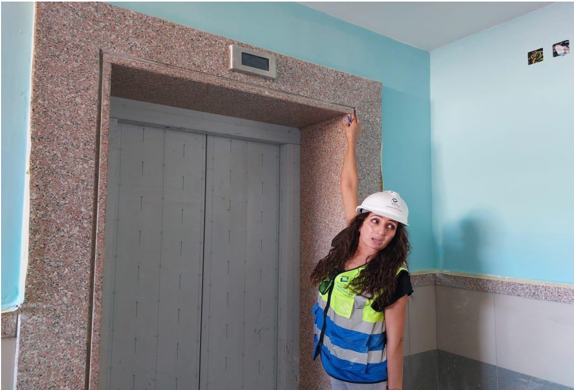
Protrusion of granite/elevator frame
