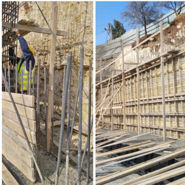
Figure #3: (a) The vertical concrete reinforcement bars that were observed to be bent for workers to pass through on site; and (b) Unsafe scaffolding and platform units on site. Photo credit: Odai Tawalbeh, 1/6/2021
