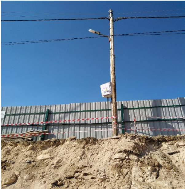
Figure #2: A power pole was observed at the top edge of excavation in unsafe condition. Photo credit: Odai Tawalbeh, 11/18/2020
