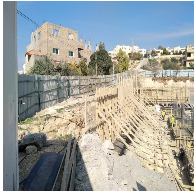
Figure #2: CORRECTIVE ACTION PLAN CLOSED – power pole removed and shoring system installed. Photo credit: Odai Tawalbeh, 1/6/2021
