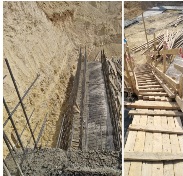
Figure #4: (a) Unguarded vertical concrete reinforcement bars that were observed on site; and (b) Unsafe access ramp on site. Photo credit: Odai Tawalbeh, 1/6/2021
