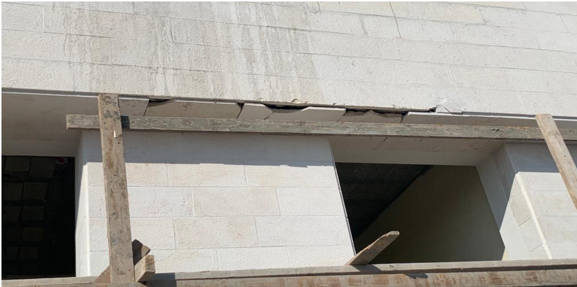
Defected stones at the facades
