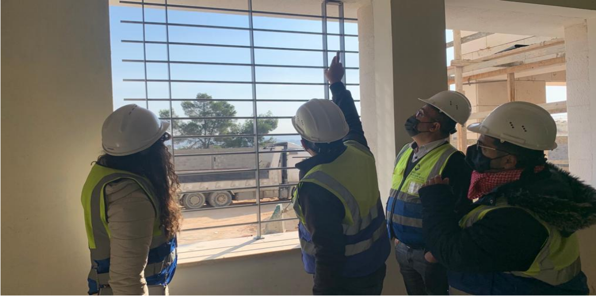
Defects in the steel protection grill
