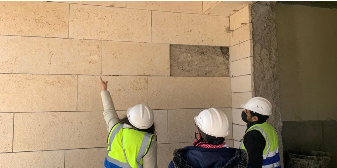
Defected stones at the facades
