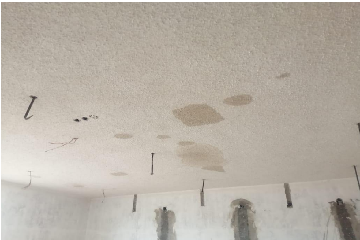
Water penetration due to defects in the waterproofing
