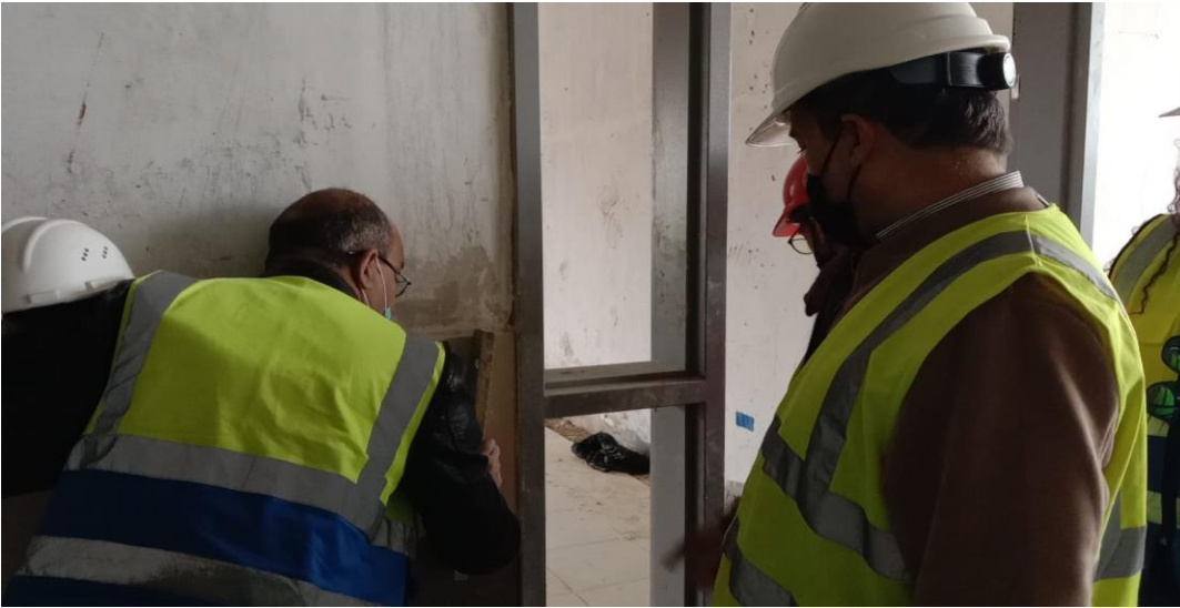
Defects in verticality of parts of porcelain wall tiles
