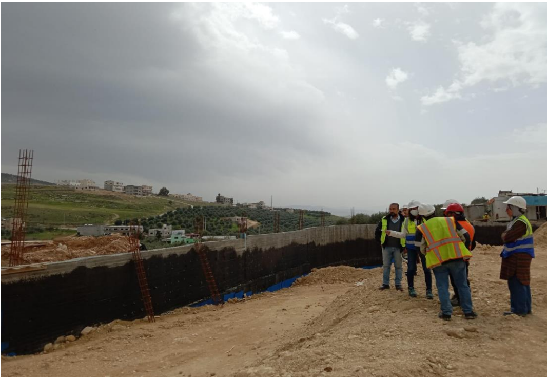
Defects in cartonal boards at boundary walls
