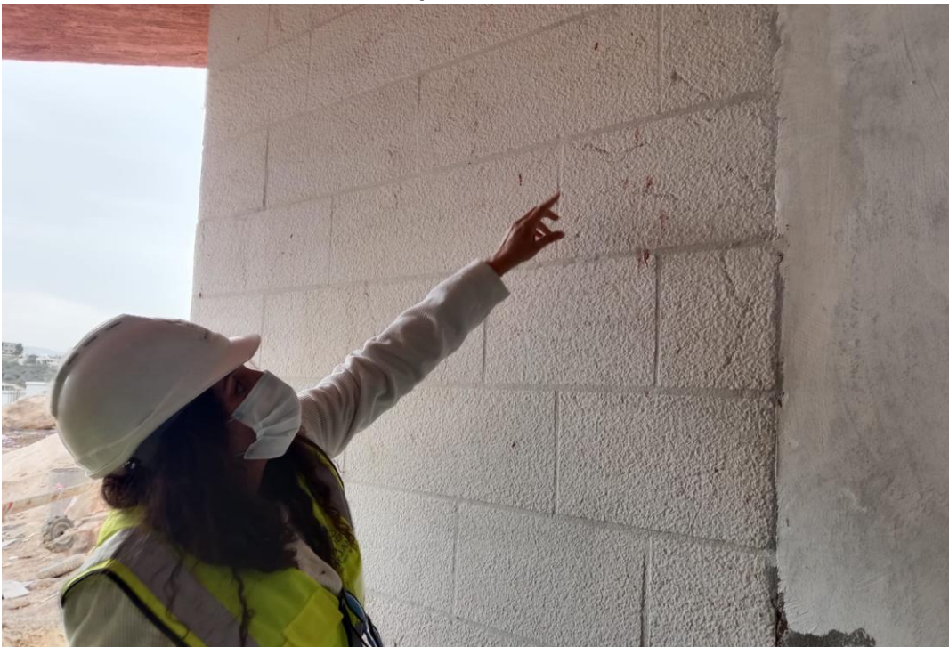
Defects in built stones at the entrance
