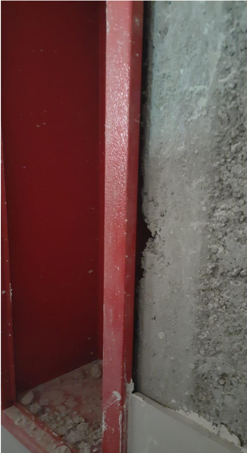
Defects in fire extinguisher cabinet
