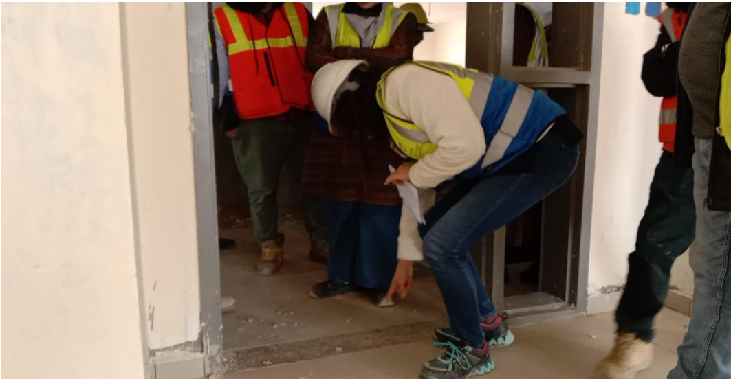
Broken and unlevelled threshold
