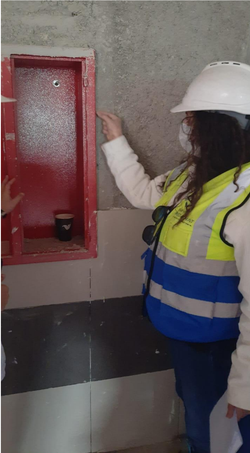
Defects in fire hose cabinet
