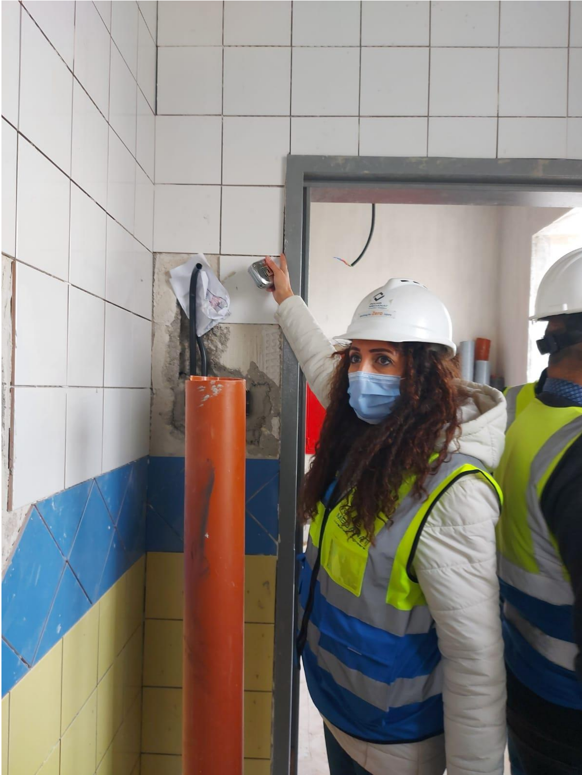
The team inspected the wall tiling at the wet areas and observed unaccepted cutting of tiles adjacent to the door frames (figure:17 & 18)
