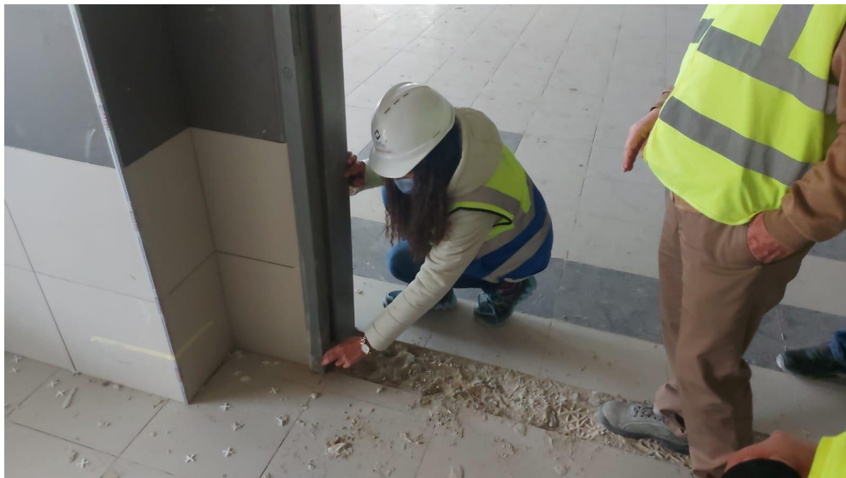
The team discussed with the Contractor the dimensions of the sill at the entrance of the multi-purpose hall
