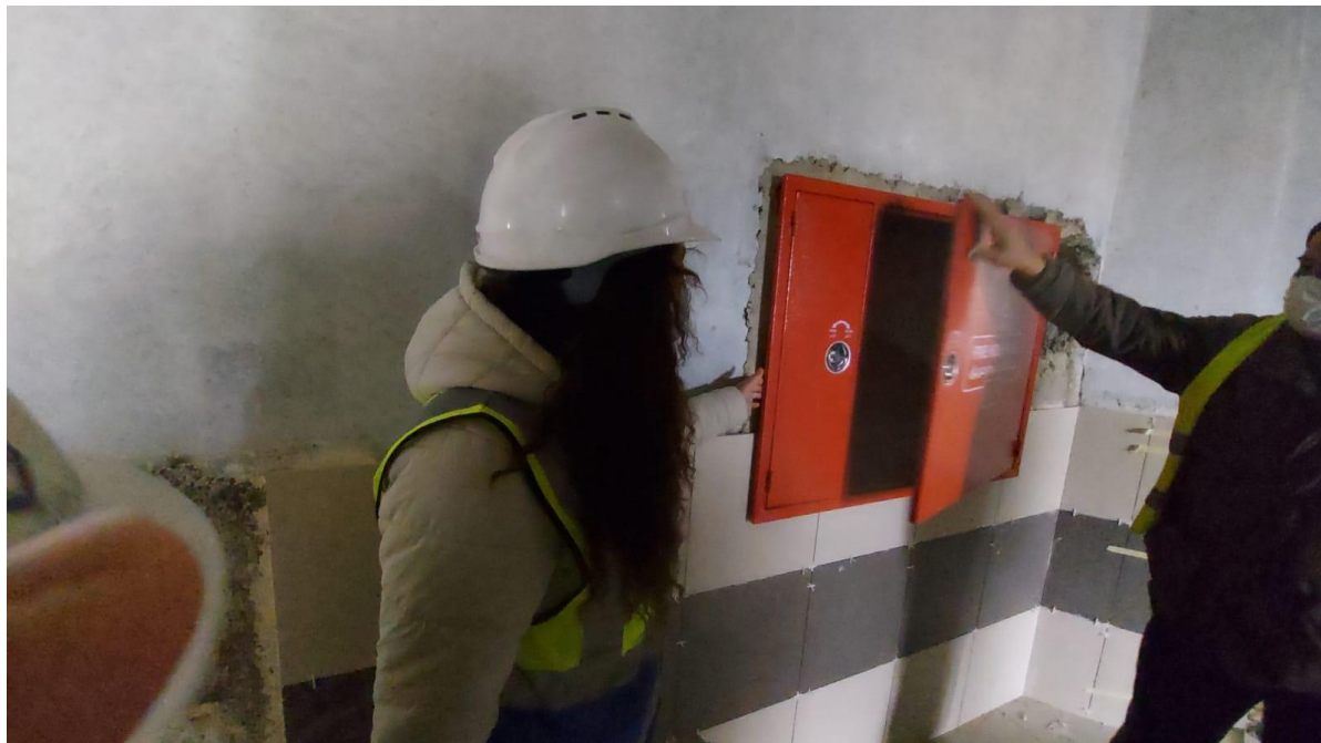
The team inspected the installation of the fire hose cabinets and requested the Contractor to submit two samples in order to choose one to be executed
