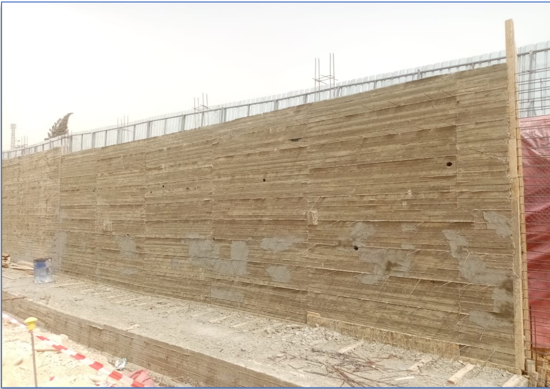
Figure 6: Segregation in Boundary Walls
