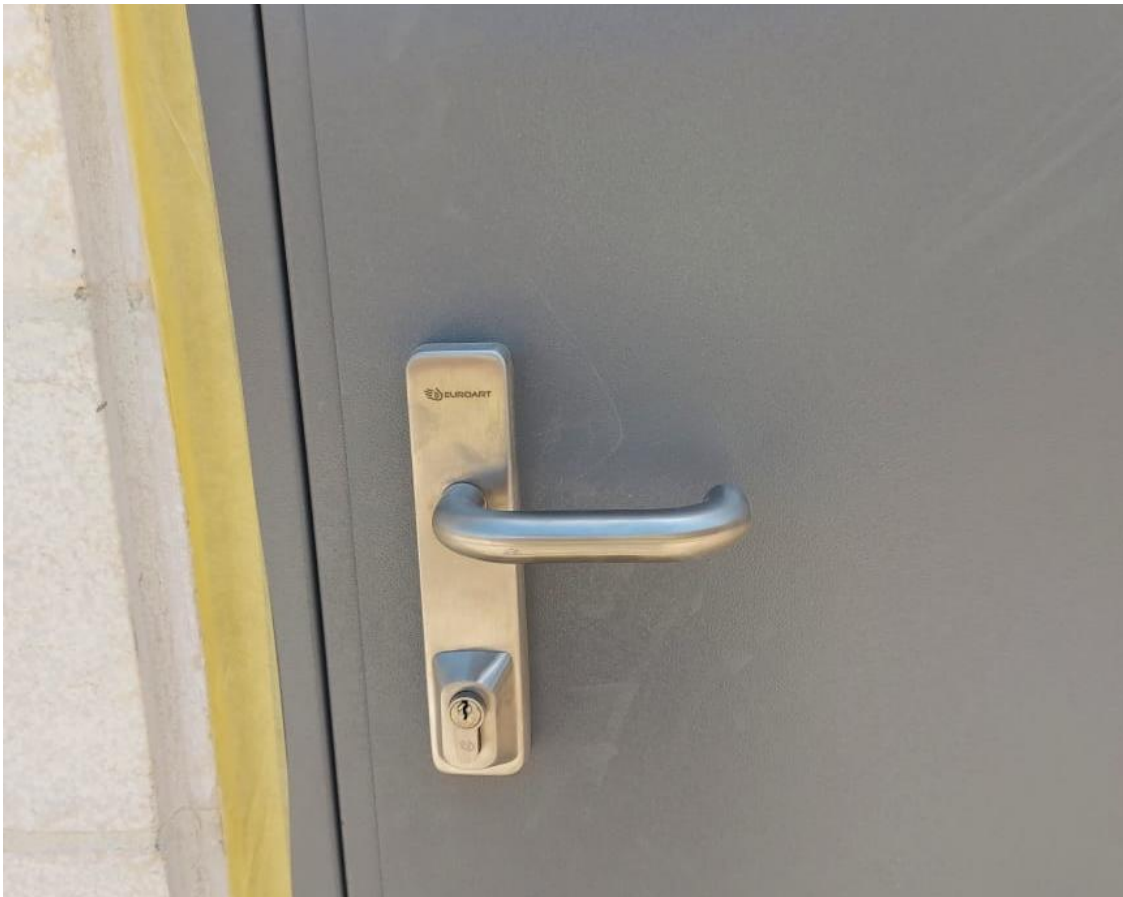
The team inspected the installation of steel doors and their accessories (figure:18 & 19)
