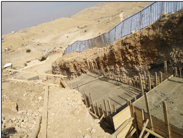
Figure #12: Lack of Lateral Support for Deep Excavations, Risk of Collapse, Serious Injuries. The area was closed by the Contractor, however, a competent person experienced in excavation work must inspect this dangerous area to assess ground conditions and determines the appropriate shoring system for the site, according to Soil Test Results. Photo credit: Odai Tawalbeh, 1/25/2021
