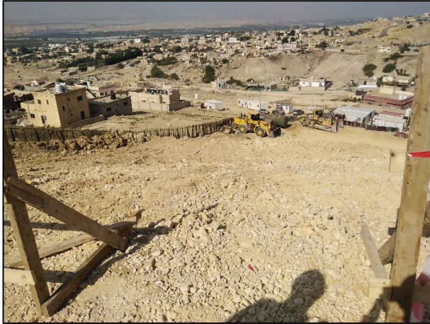
Figure #11: An Effective Guardrail Edge Protection System should be Installed on Site. Photo credit: Odai Tawalbeh, 1/25/2021
