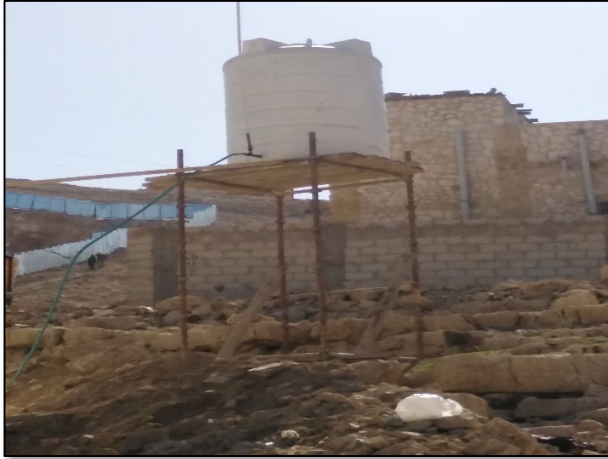
Figure #5: A Water Tank Placed on Unsafe Scaffold. Photo credit: Odai Tawalbeh, 1/25/2021
