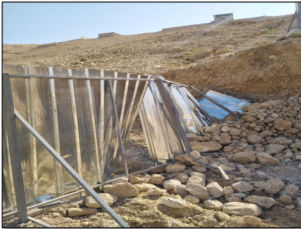
Figure #9: Part of the Temporary fencing was Damaged as a result of Collapsing Soil & Rocks near it on Site. Photo credit: Odai Tawalbeh, 1/25/2021
