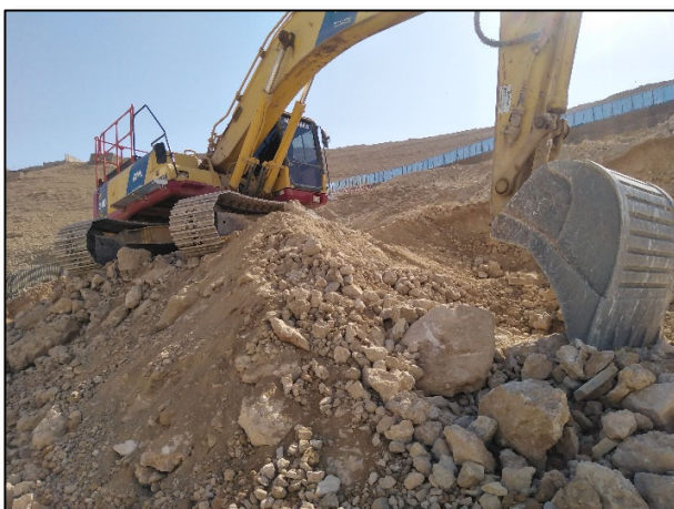
Figure #13: This Excavator Located at the Edge of An Unbelievable Slope in An Extremely Scary Conditions. Immediate Corrective Action had been Taken. However, REMEMBER: Precautions Must ALWAYS Be Taken in Mountain Regions, AND Operators Really Need To Develop A Feel For The Controls When Digging On A Slope. Photo credit: Odai Tawalbeh, 1/25/2021
