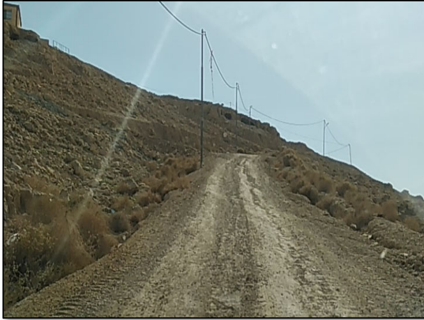
Figure #8: Gravel Road for Site Equipment & Vehicles – No Barriers, Warning Tapes, Warning Signs and Speed Limit Signs were observed along the road leading to the site. Photo credit: Odai Tawalbeh, 1/25/2021
