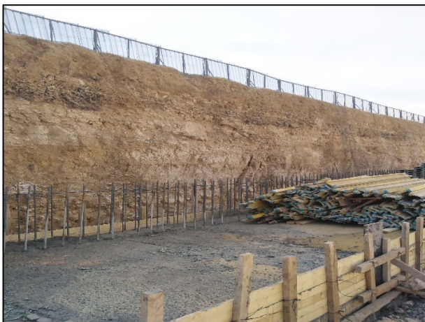
Figure #10: Rockfall Protection Steel Wire Mesh has been installed, however, a competent person experienced in excavation work must inspect this area to assess whether this support is sufficient or not. Photo credit: Odai Tawalbeh, 1/25/2021
