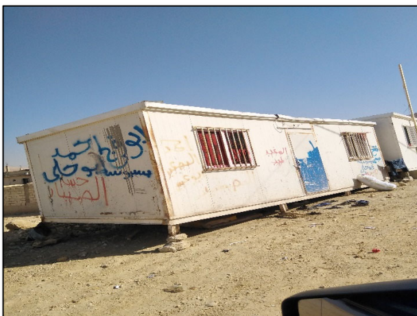
Figure #4: Unsafe Contractor Office Trailers, fixed on unstable objects. Photo credit: Odai Tawalbeh, 1/25/2021
