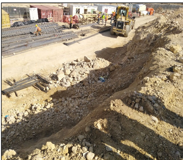
Figure #7: Movement of Heavy Equipment very close to the Excavated Portion and Lack of Lateral Support may lead to the Collapse of Soil and Rocks from the top of the Slope towards the Site Offices, which may result in Serious Injuries. We've already recommended the assigned Contractor to install an additional temporary support along the site offices and the immediate corrective action has been taken by the next day of our site visit. Accordingly, we will arrange another field trip ASAP to re-inspect the site and ensure that the required support is effective. Photo credit: Odai Tawalbeh, 1/25/2021
