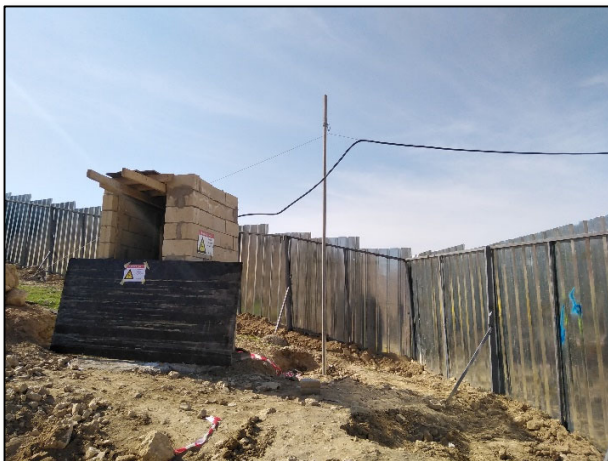
Figure #6: The Roof of Temporary Electrical Room was Not Properly Protected from the Rain, It will be A Real Hazard if Rainstorm Hit the Site. Photo credit: Odai Tawalbeh, 1/25/2021
