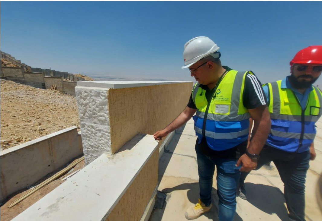
Broken stone coping
