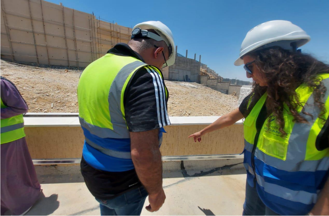
The parapet plastering is not compatible with flashing
