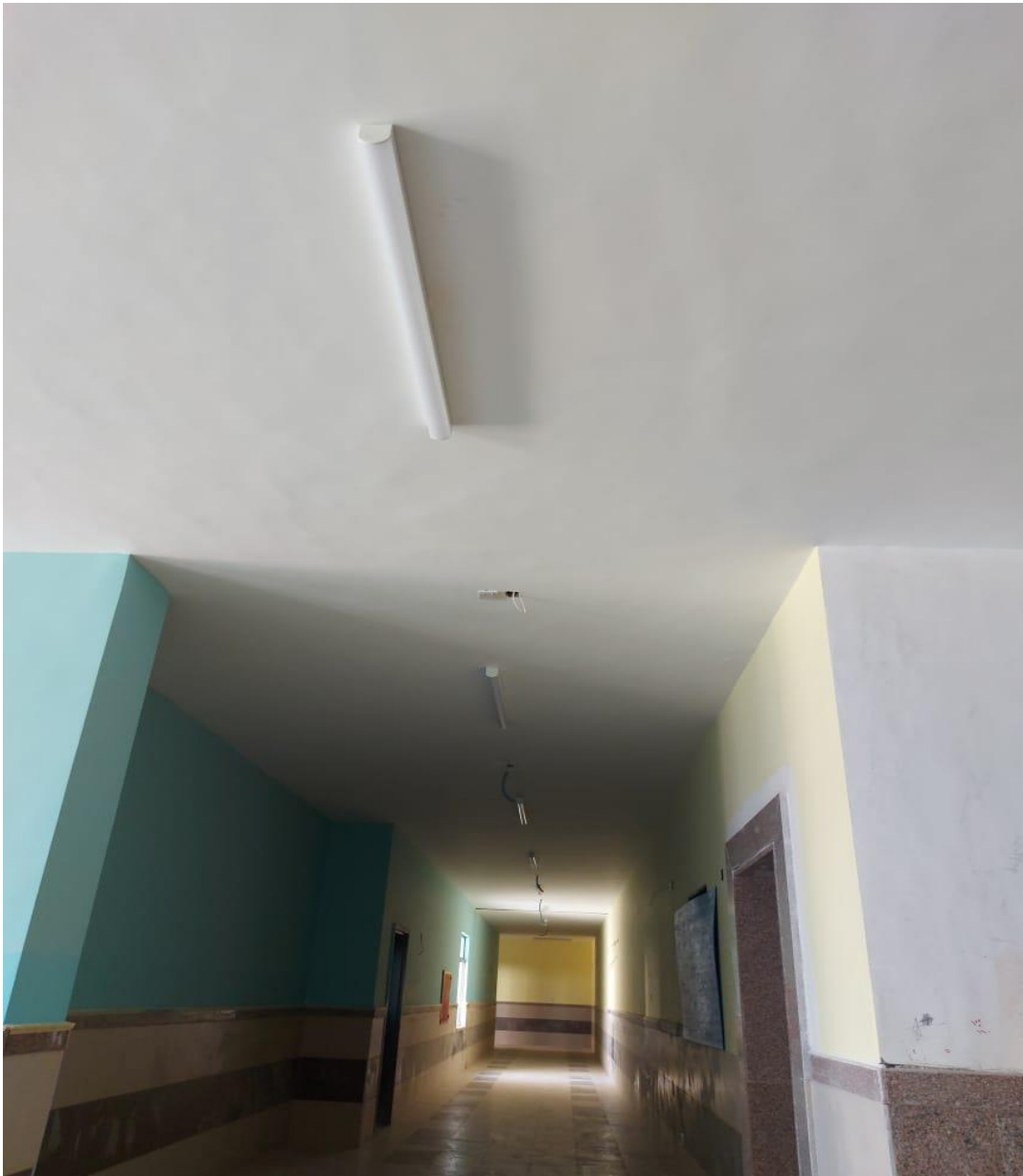
Waving in plastering of ceiling
