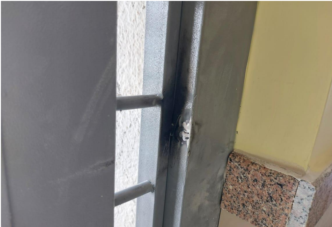
Defects in the installation of steel doors at the entrance
