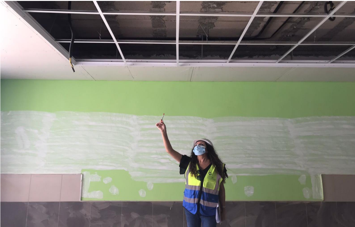
Hangers holding suspended ceiling are not vertical
