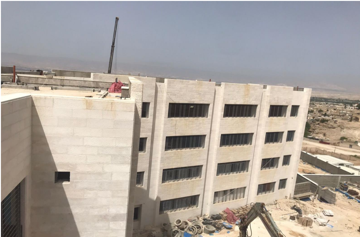
Dirt at the stone facades
