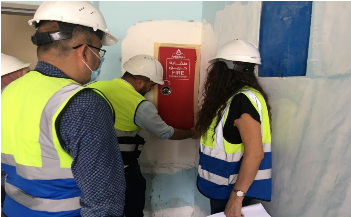
Gap between the cabinets and the wall
