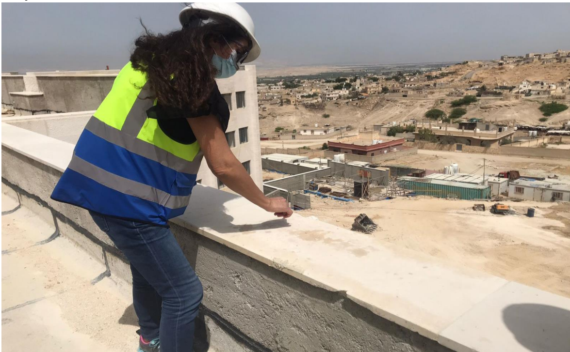
Broken stone coping
