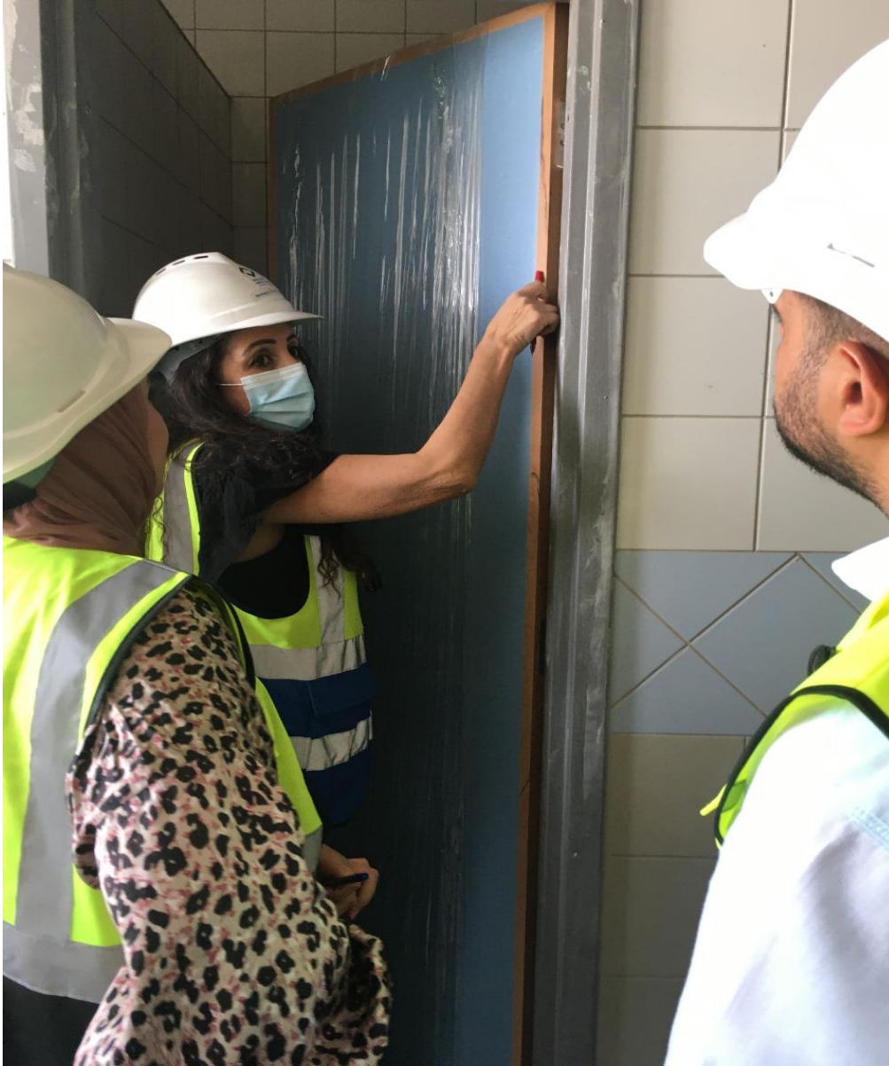
Defects in beech wood frame
