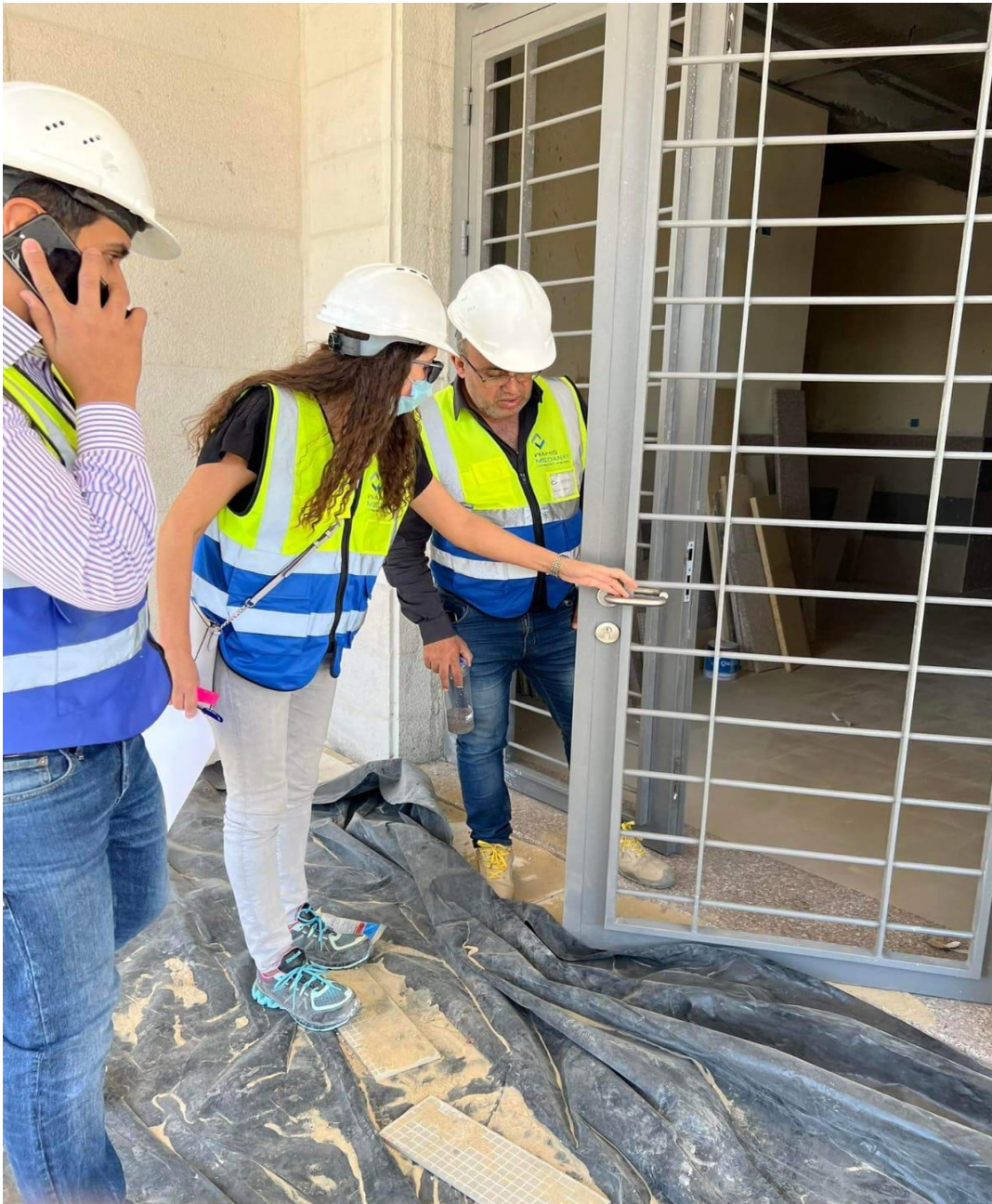
Defects in the main steel doors
