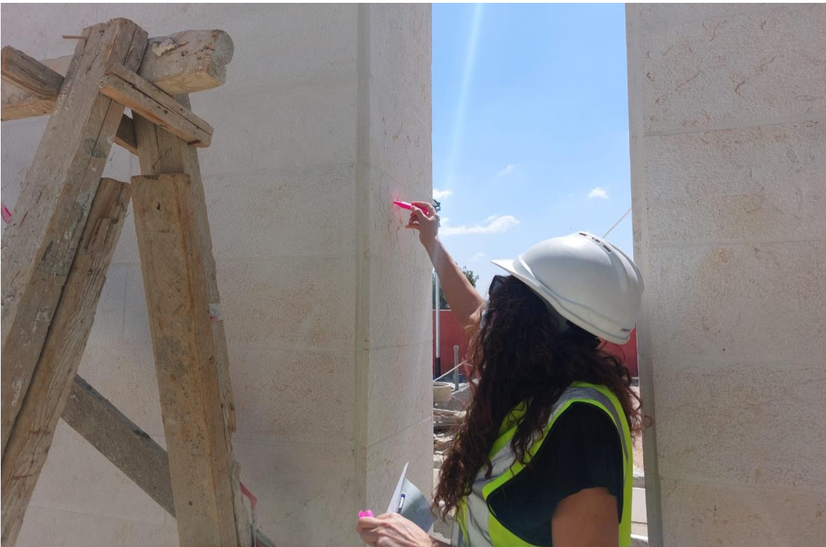
Defects in the built stones
