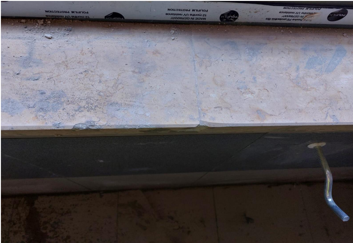
Broken window sill
