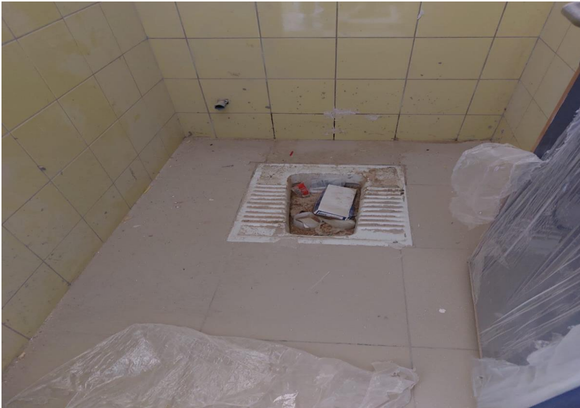
Accumulated debris and dirt at the sanitary fixtures
