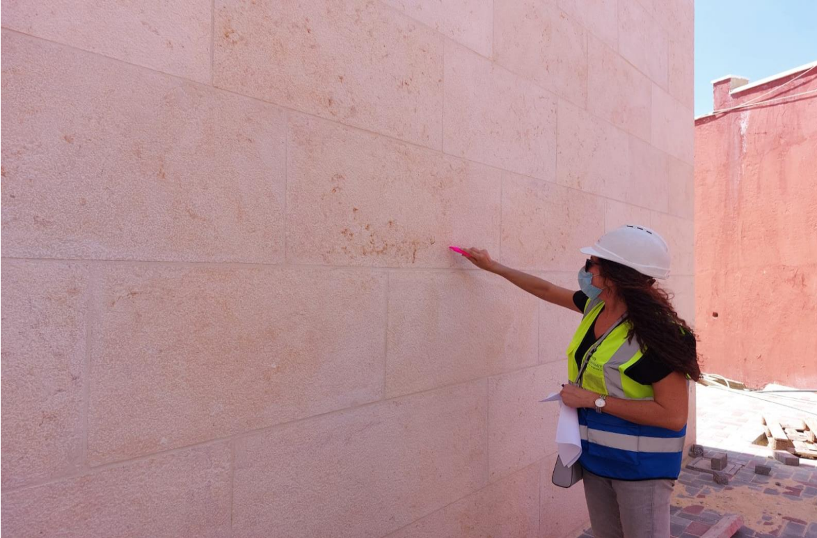
Defects in the built stones
