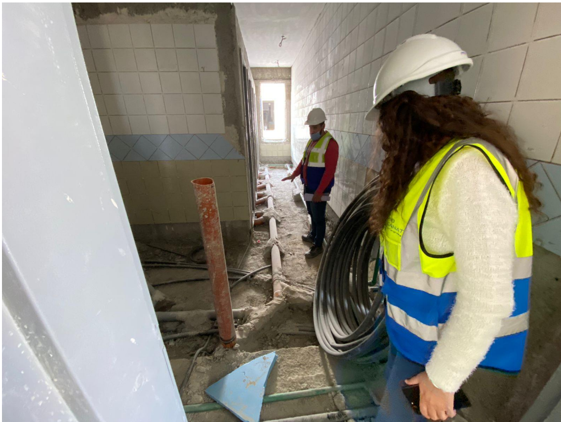
The team conducted general inspection to the water supply and drainage networks inside the wet areas
