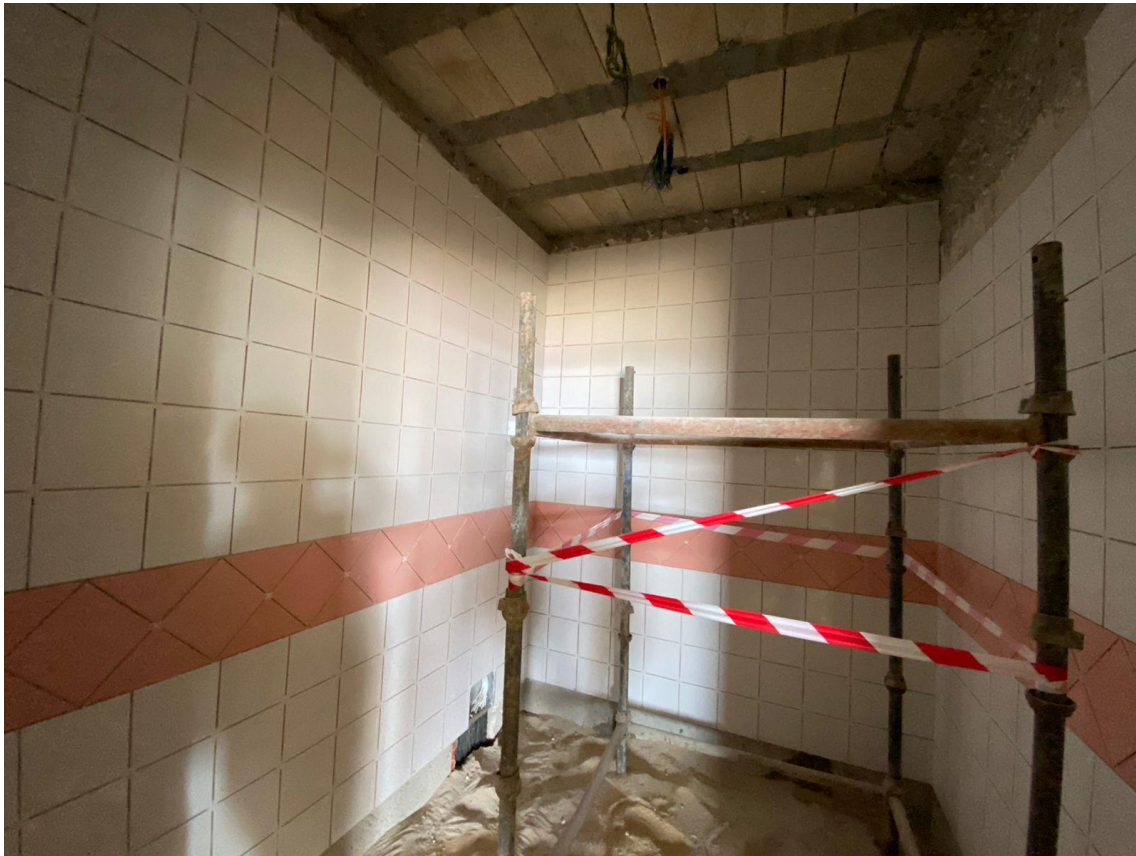
The supervision team inspected the executed works for the ceramic wall tiles at the wet areas
