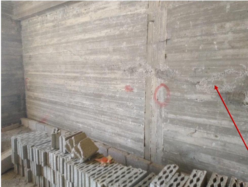
FIGURE #11 & 12: Roughness and segregation in concrete was noticed on walls
