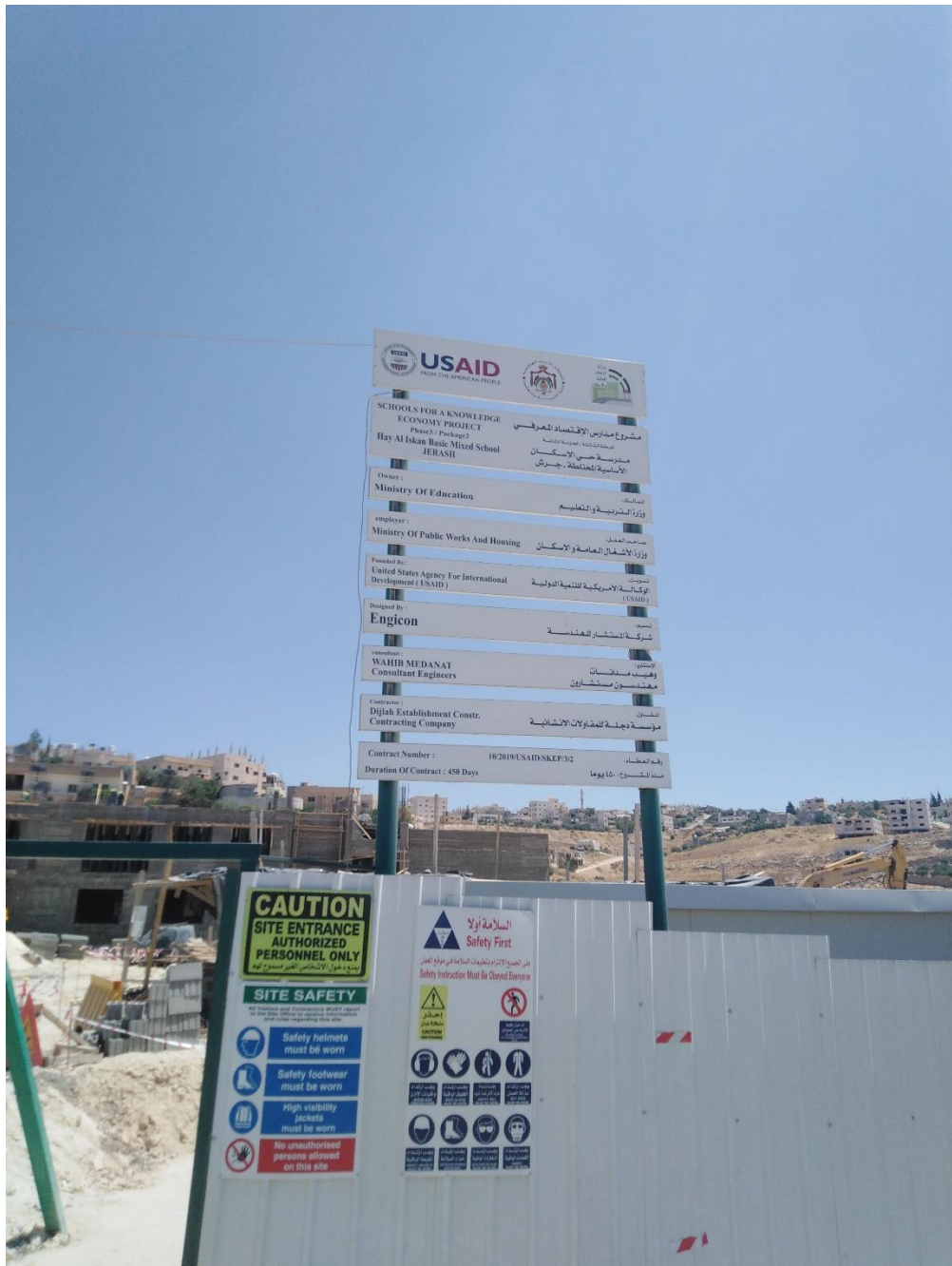
FIGURE #01: Project ID Sign on site. Photo credit: Osama Obeid CMTO/Trigon May 23,, 2021
