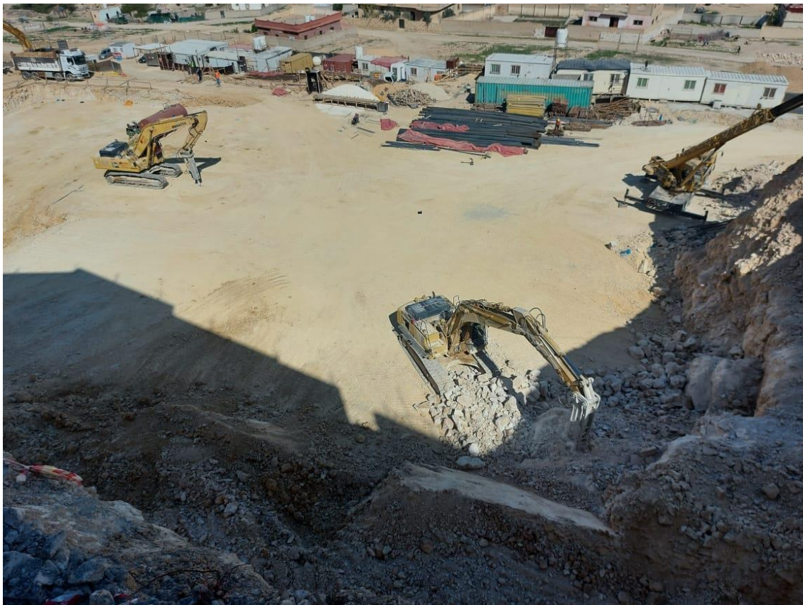
Main building excavation work continued in accordance to designer recommendation - original design drawings
