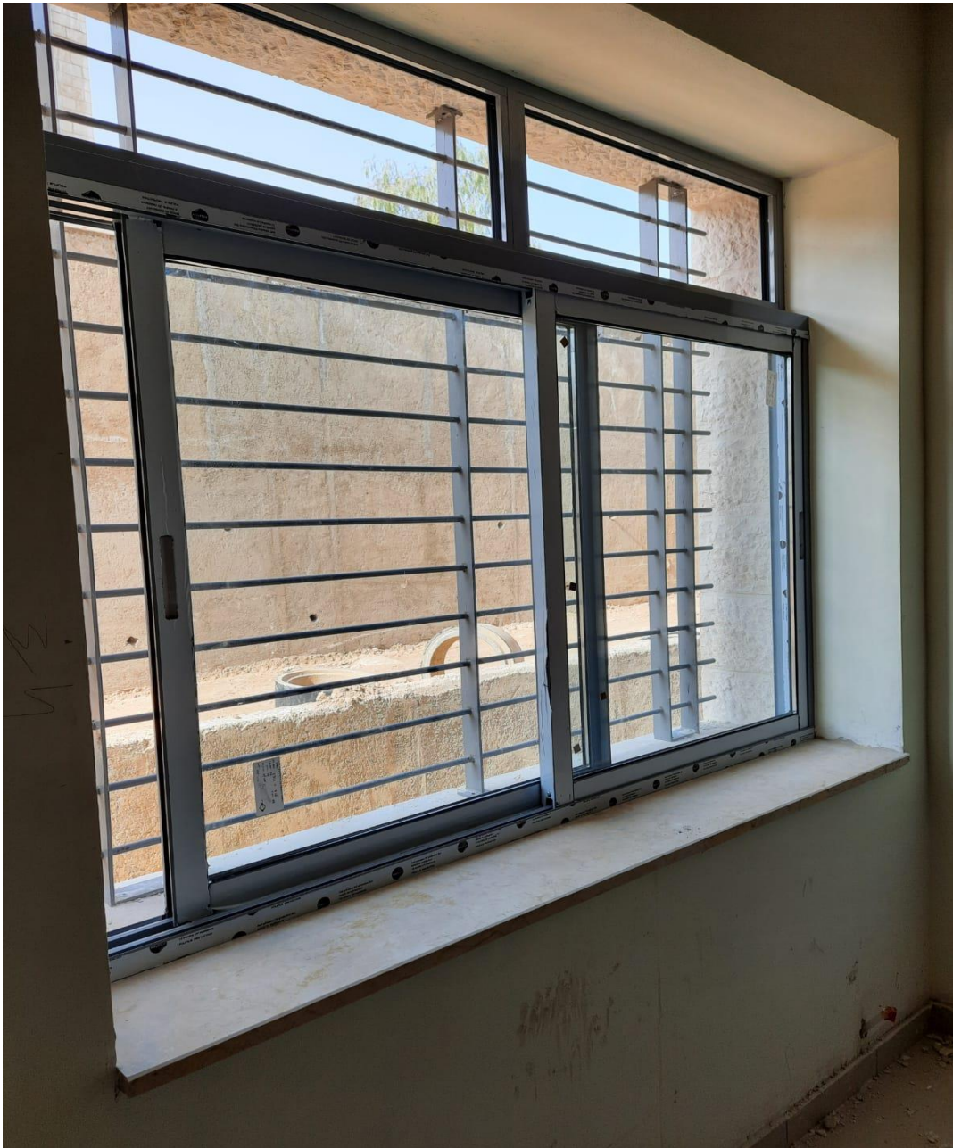
Defects in installed aluminum window
