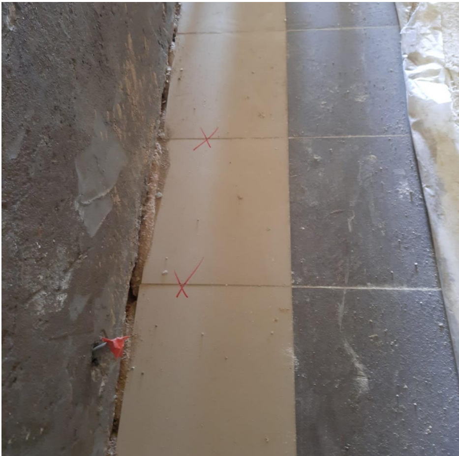
Teething at the porcelain floor tiles at the corridor
