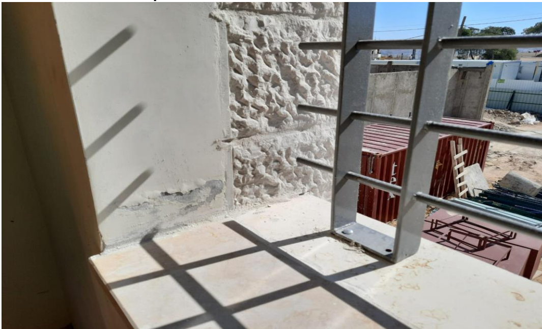
Defect at the window jamb
