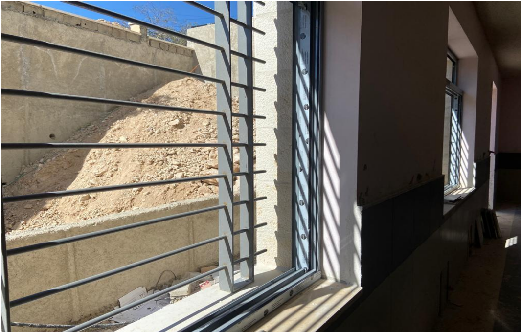
Corrosion at the steel protection screen
