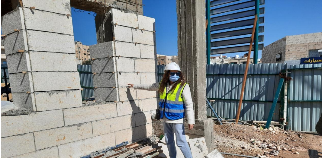
Defected stones at the guard room
