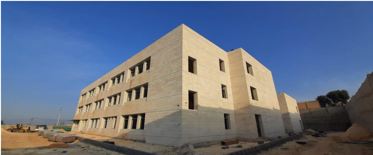
Base course at the walkways not conforming to the requirements
