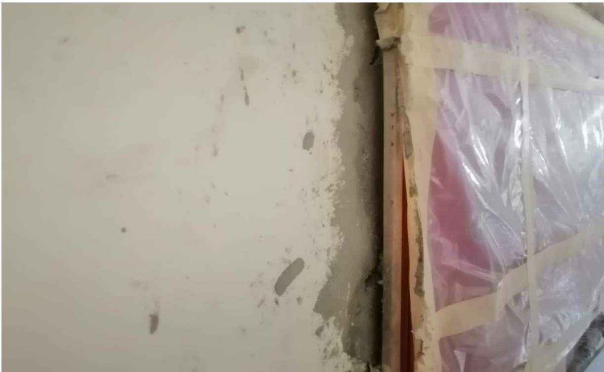
Gap between the cabinets and the wall
