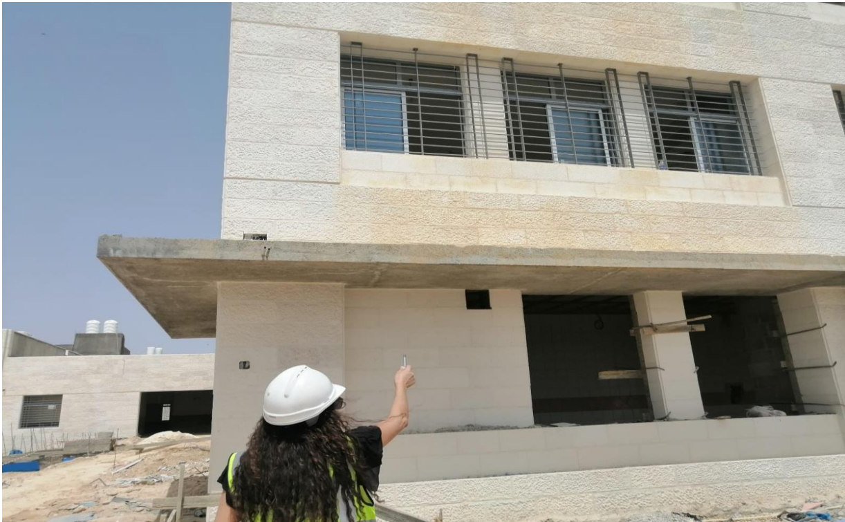
Defected stones and dirt
