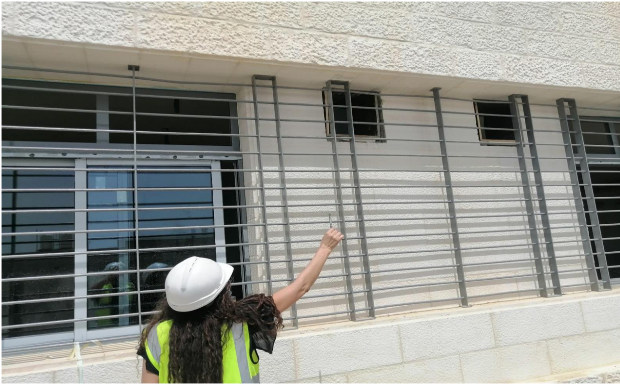
Unrepaired steel protection screens
