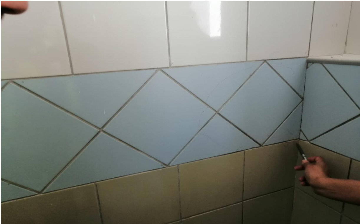
Broken ceramic wall tiles
