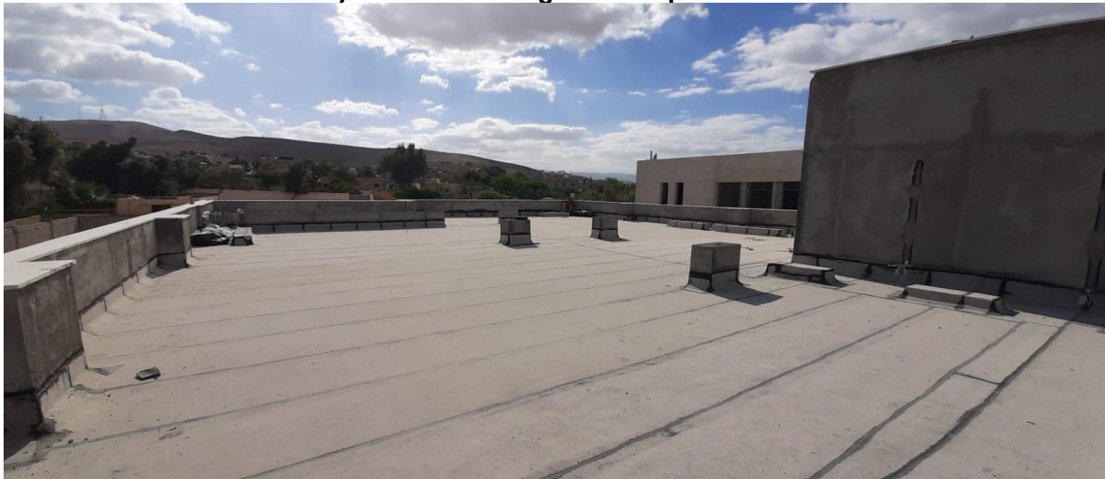
Defects in sheet waterproofing
