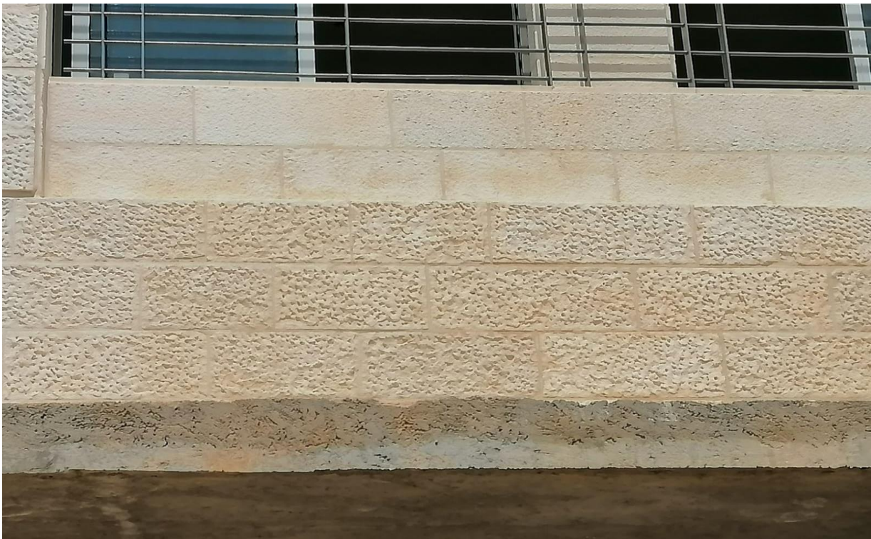
Defected stones and dirt
