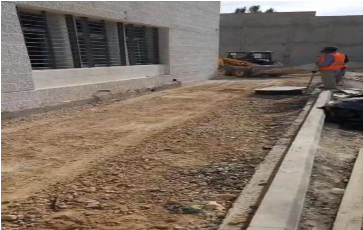
Removal of base course not conforming to the requirements
