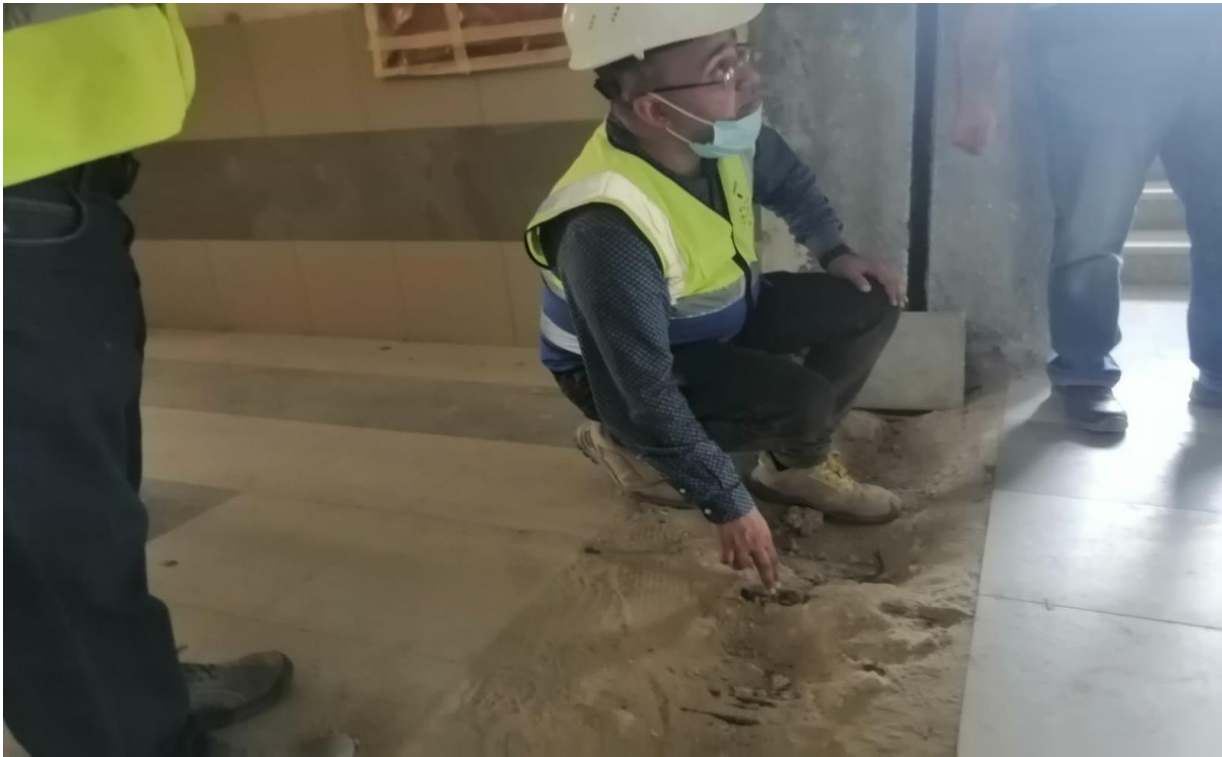
The level of conduit contradicts with tiling
