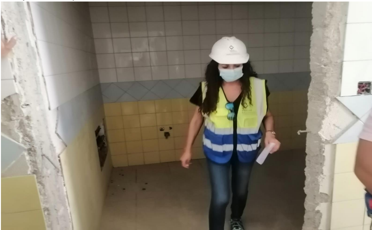
Broken ceramic wall tiles
