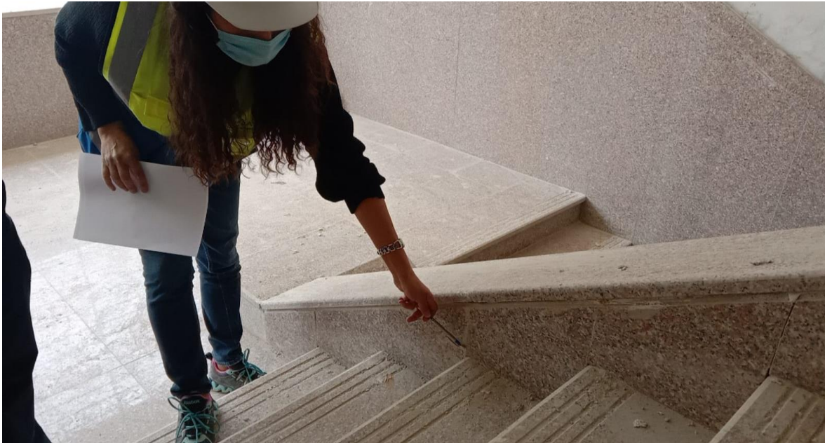
Gaps between granite pieces appeared
