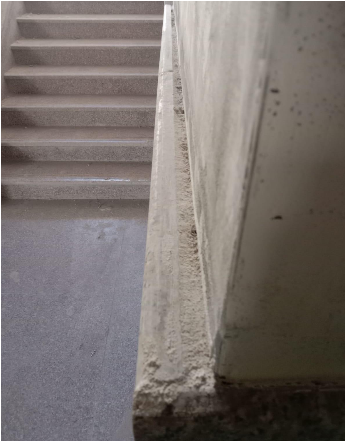
Defects in installation of granite coping
