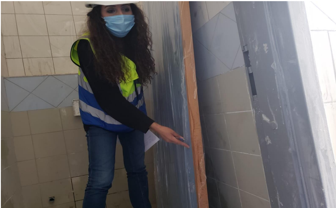
Defected wooden door frames
