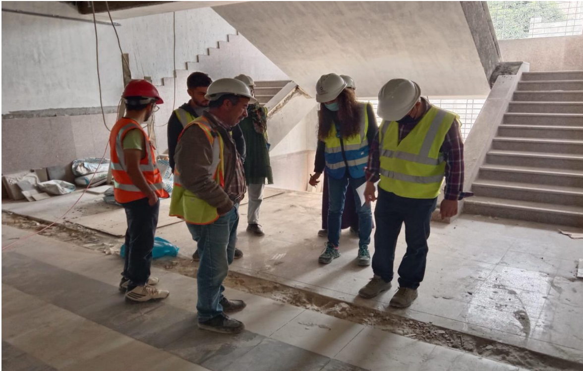
Defects in connection line between porcelain and granite
