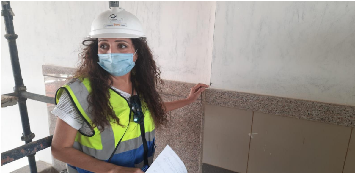
Defects in granite coping installation
