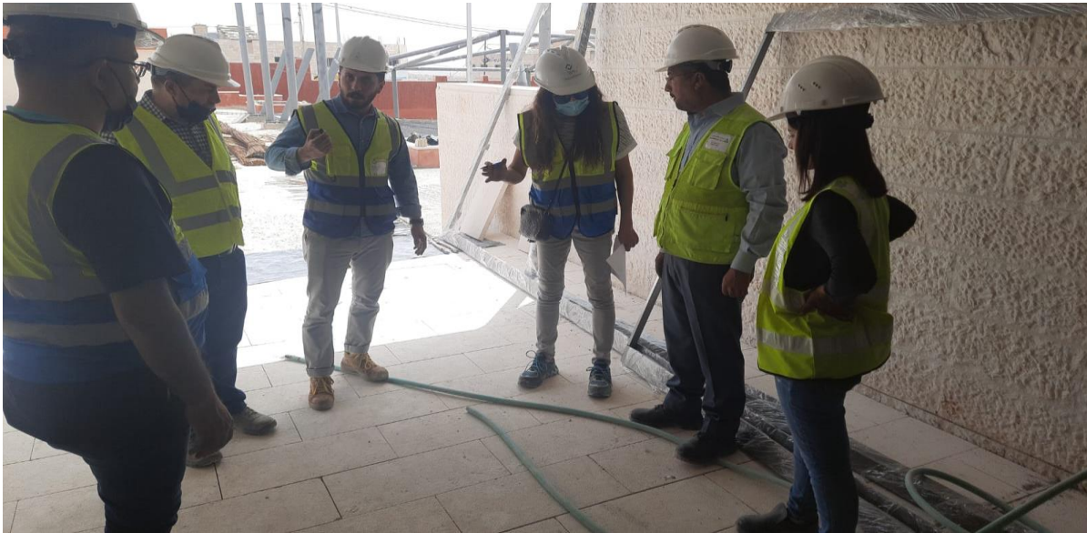
Broken stones at the entrance floor
