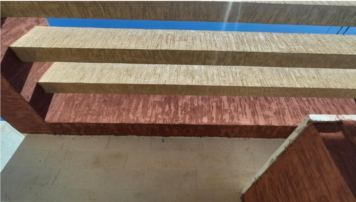
Defects in the texture of colored plastering
