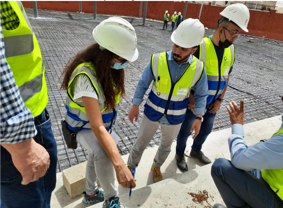
Voids at the surface of the amphitheater seats
