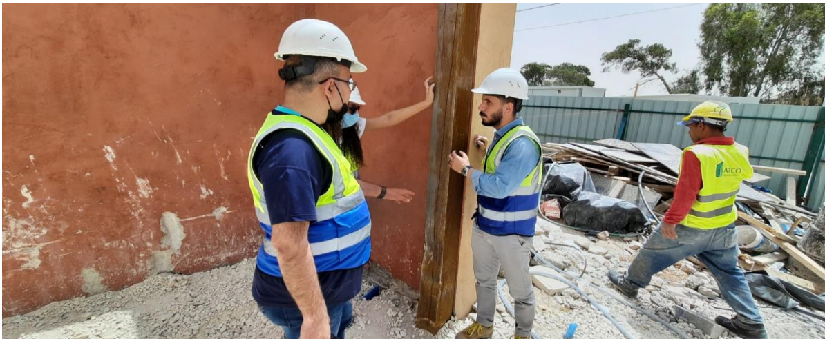
Dirt at the colored plastering
