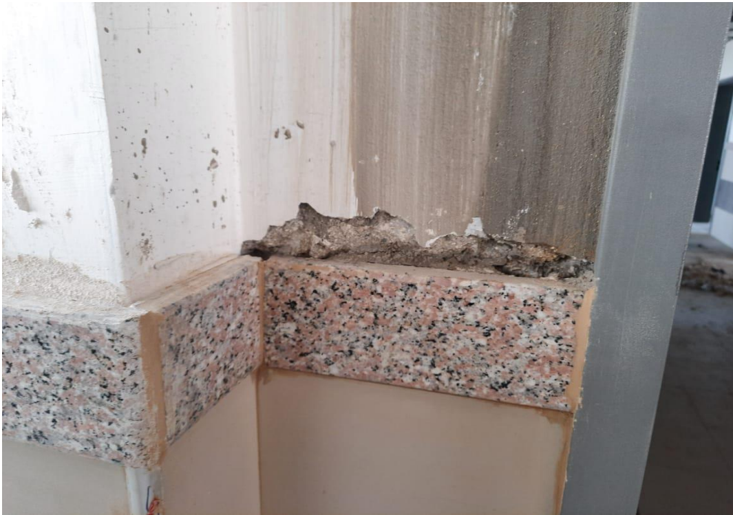
Defects in granite coping
