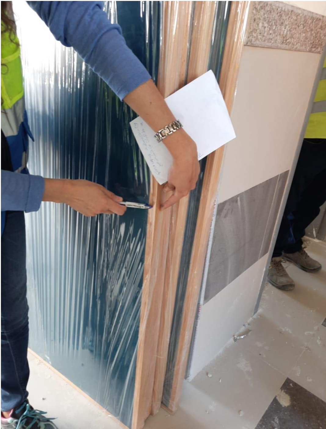
Defects in beech wood frame
