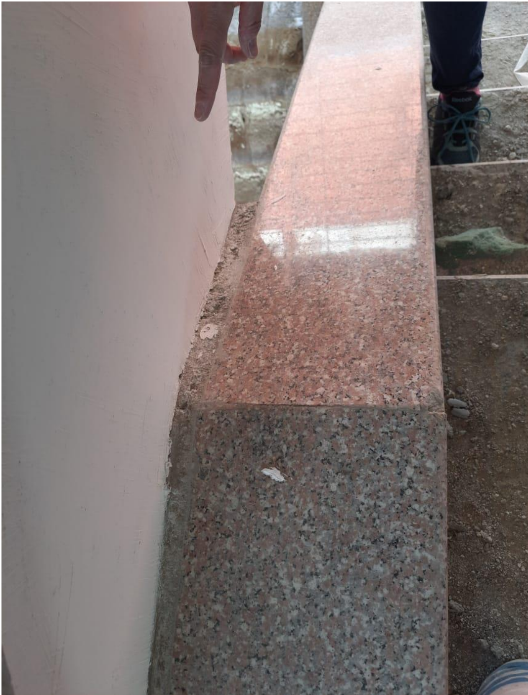
Defects in tiling
