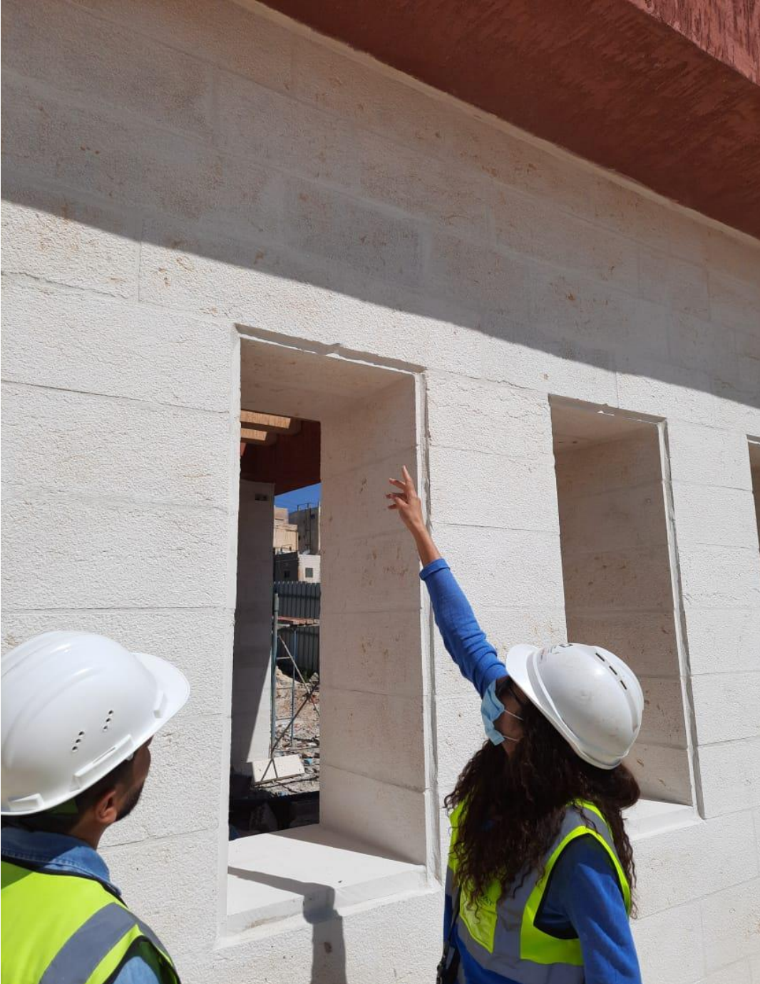
Defected stones at guard house
