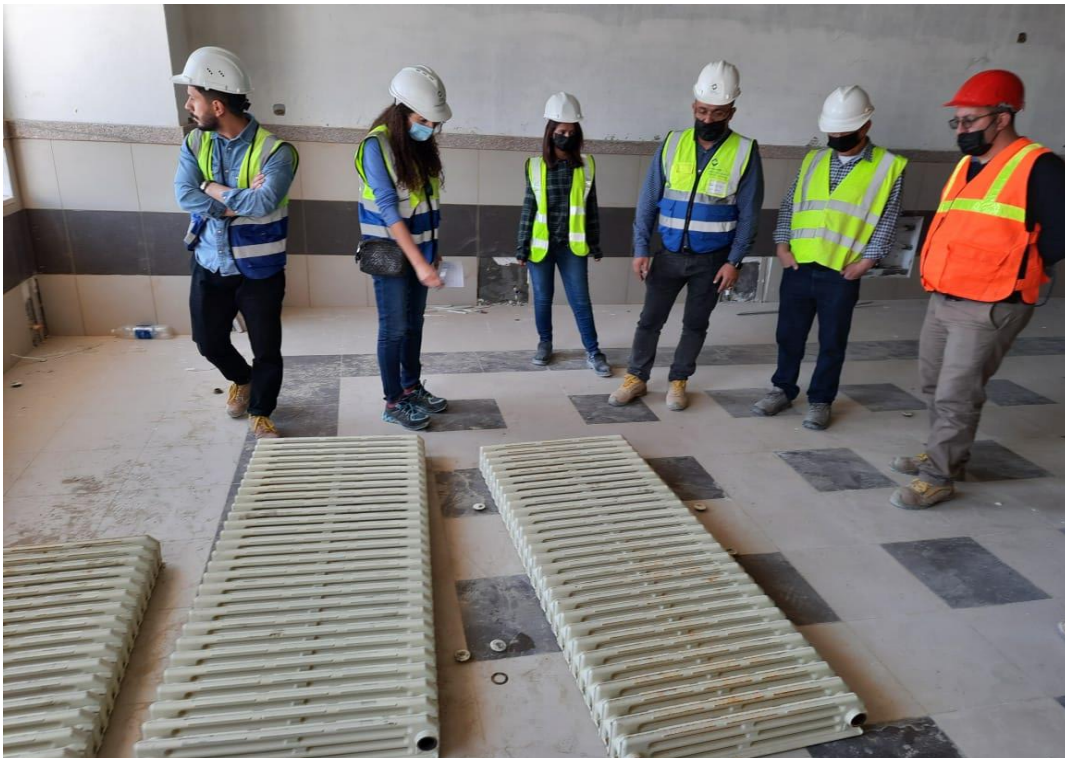
Scattered radiators on the floor tiles
