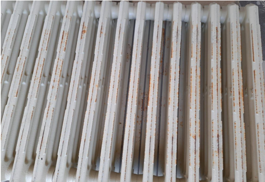
Corrosion observed on the radiators
