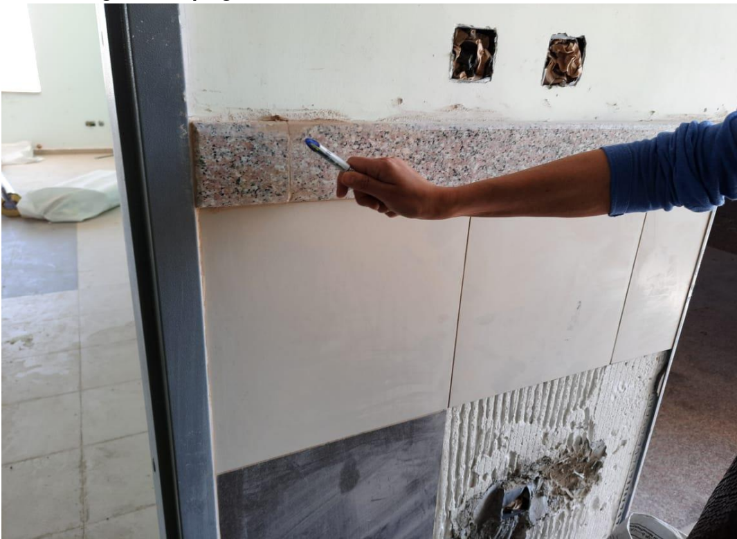
Defects in granite coping
