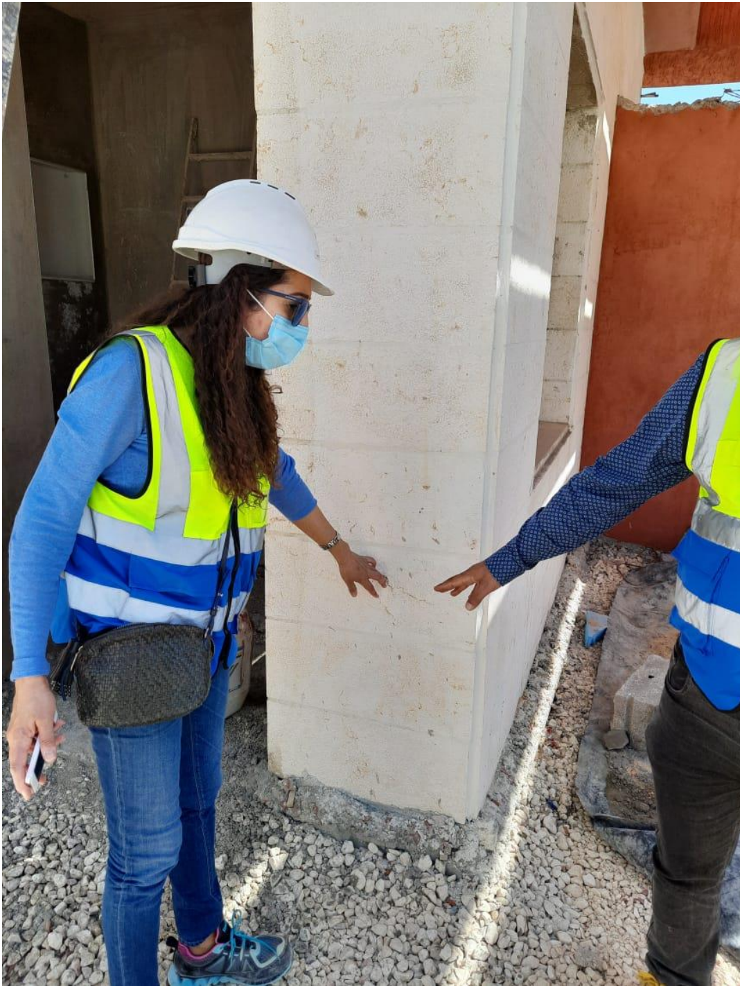
Defected stone at the guard house
