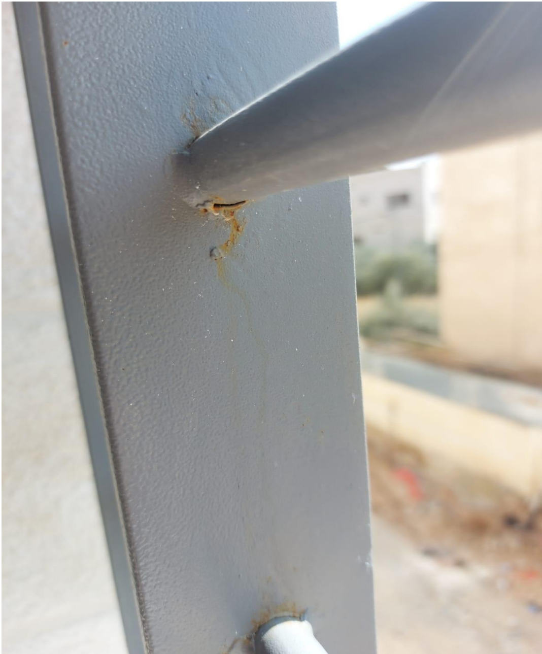
Corrosion in the steel protection screens
