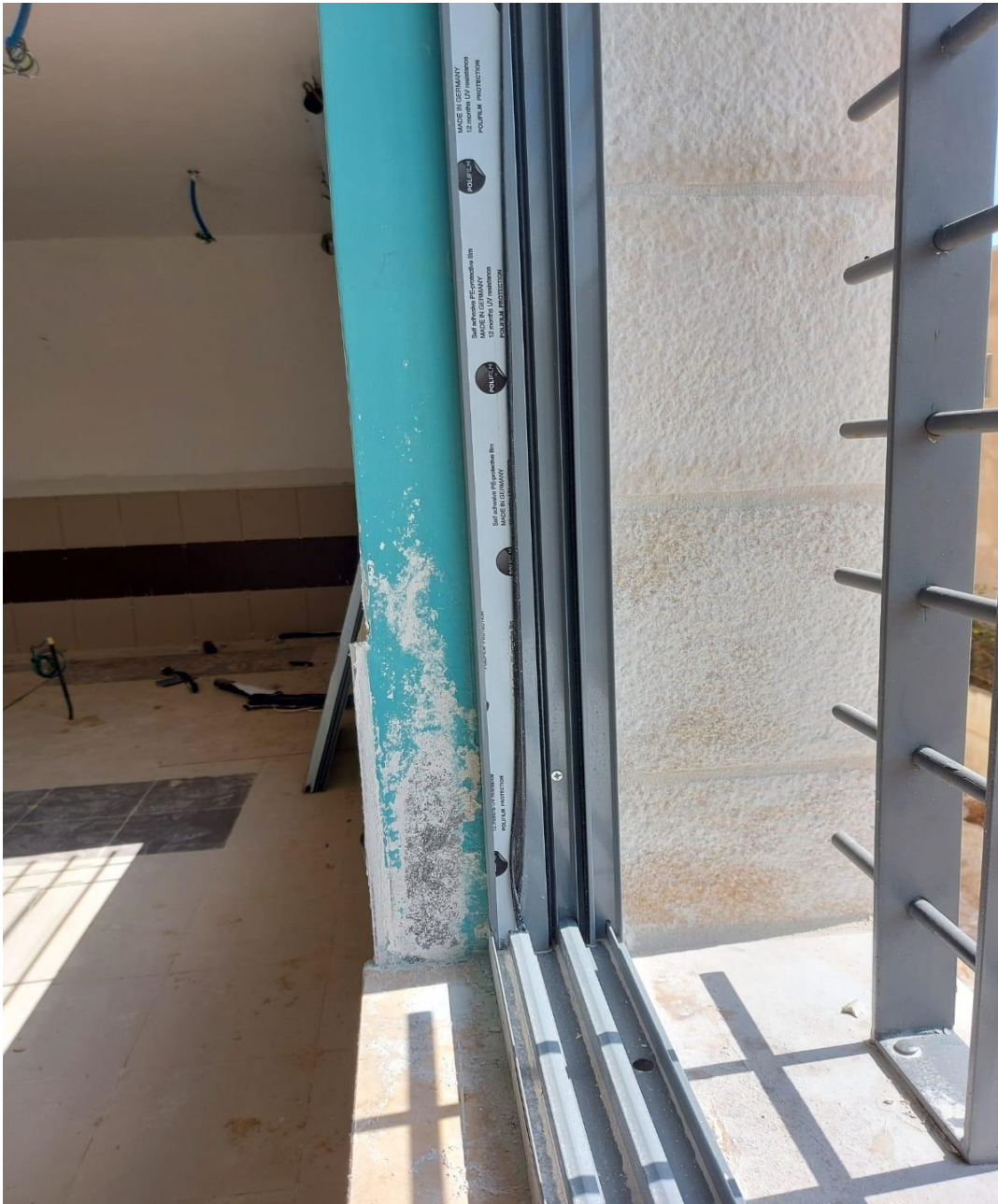
Window jambs not finished to receive aluminum sections
