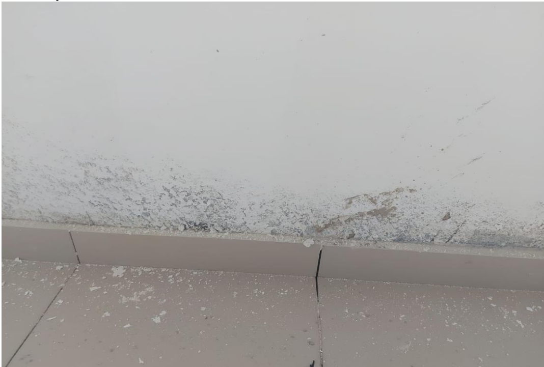
Humidity over the skirting
