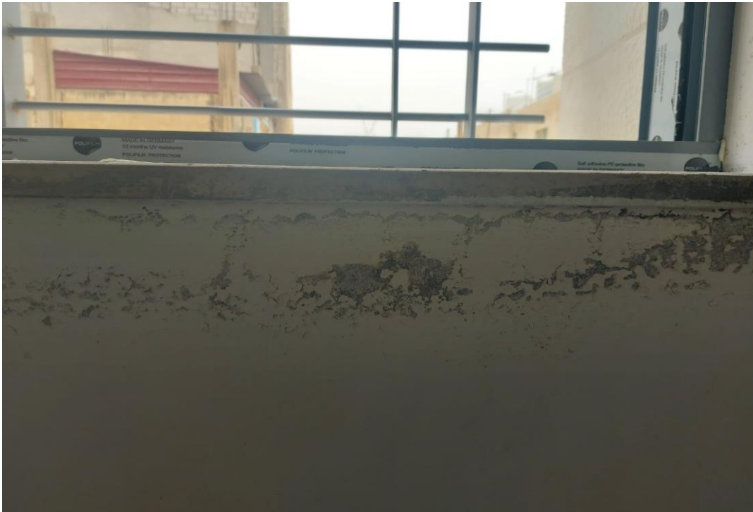
Humidity under the window sill
