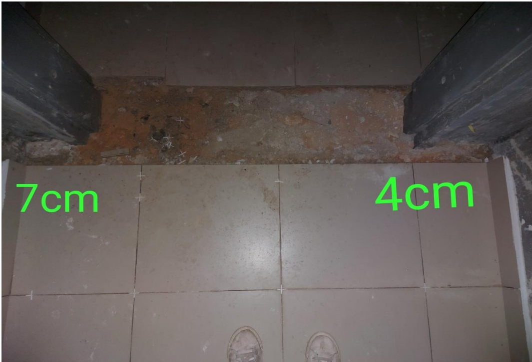
Deviation in the tiled corridor
