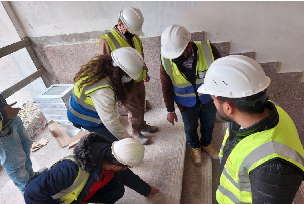
Broken staircase tread
