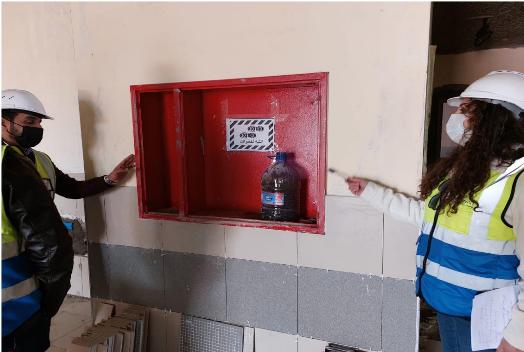
Defects in installing of fire hose cabinet
