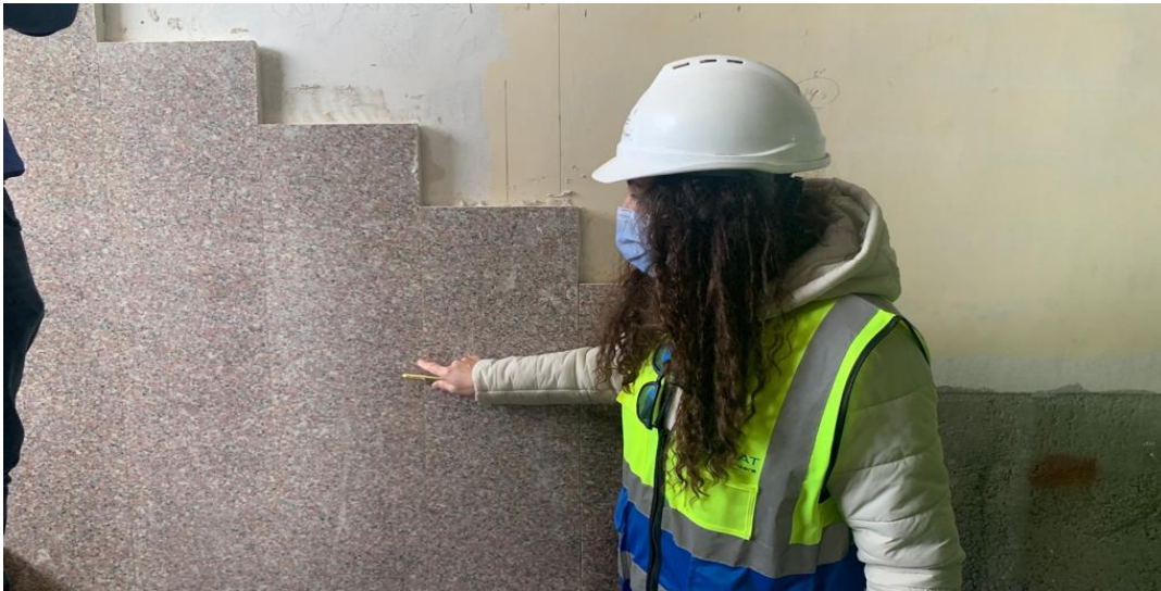
Defects in granite cladding for staircase
