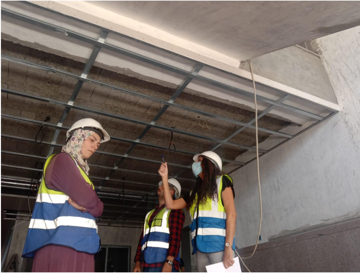
The team inspected the executed suspended ceiling and the relation with the drop beam at the staircase area
