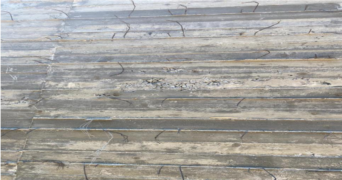
Segregation in Retaining Wall- QC Report 1304
