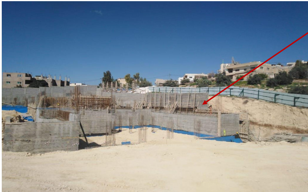
FIGURE #05: North-East side of the boundary wall is 90% completed. Photo credit: Osama Obeid Feb 9, 2021
