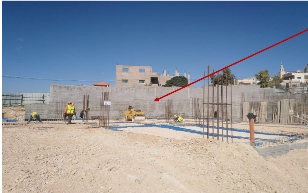
FIGURE #04: North-West side of the boundary wall is completed. Photo credit: Osama Obeid Feb 9, 2021
