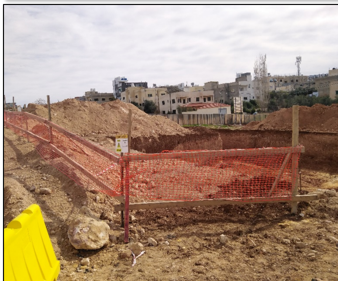
Figure #4: Excavated materials were accumulated on site – waiting for the results from RSS, to disposal or keep it. Photo credit: Odai Tawalbeh, 1/17/2021
