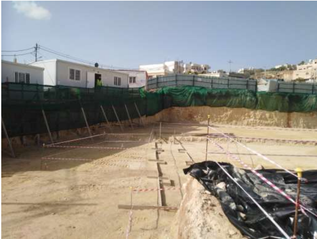
FIGURE # 06 & 07: Site offices must be Protected and supported properly from soil sliding
