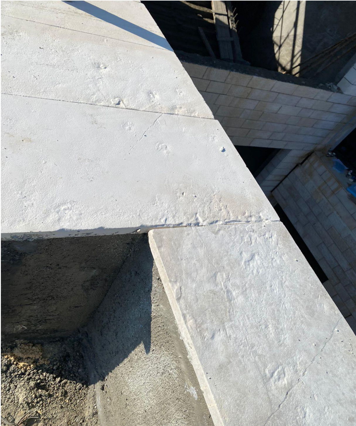
Defected stone coping
