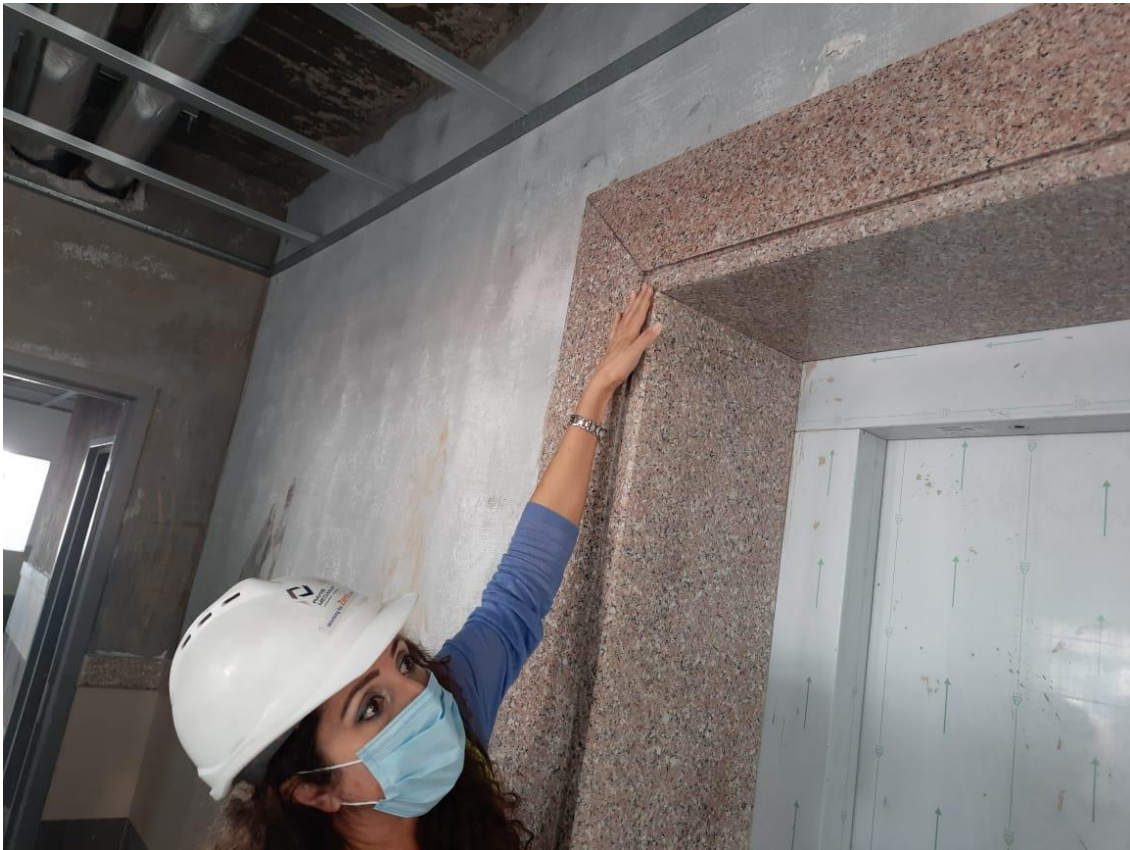
The team inspected the installed granite frame around the elevator's door and informed the Contractor with some minor remarks
