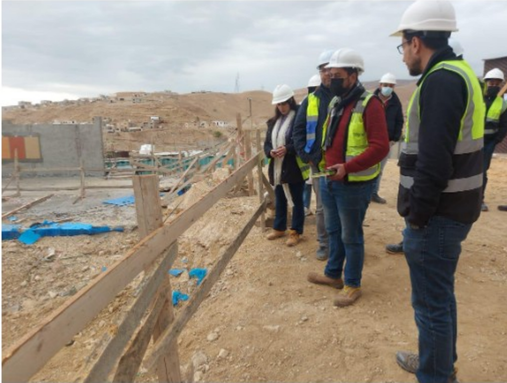
Eng. Odai pressing on the matter of installing and fixing temporary boards around excavations
