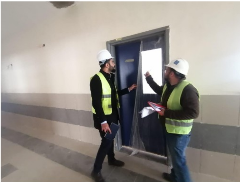
Inspecting wooden doors installation and recommending keeping them protected with the plastic covers
