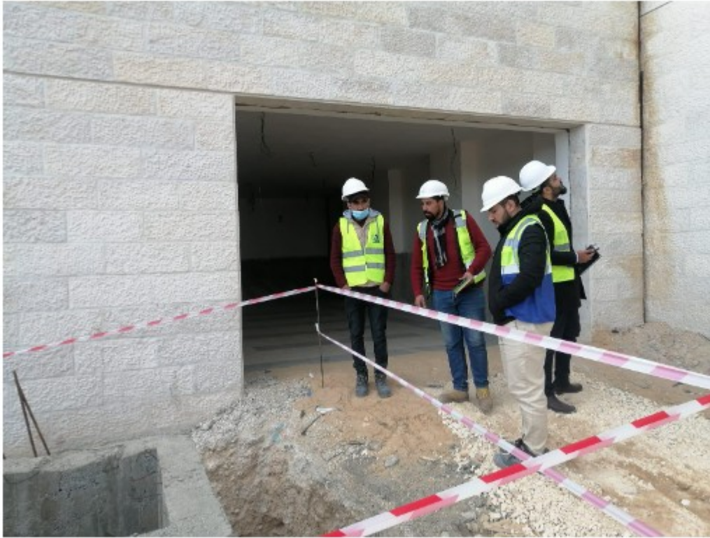
Eng. Odai instructing to put blocks or protection boards around the excavations to ensure the safety of labours
