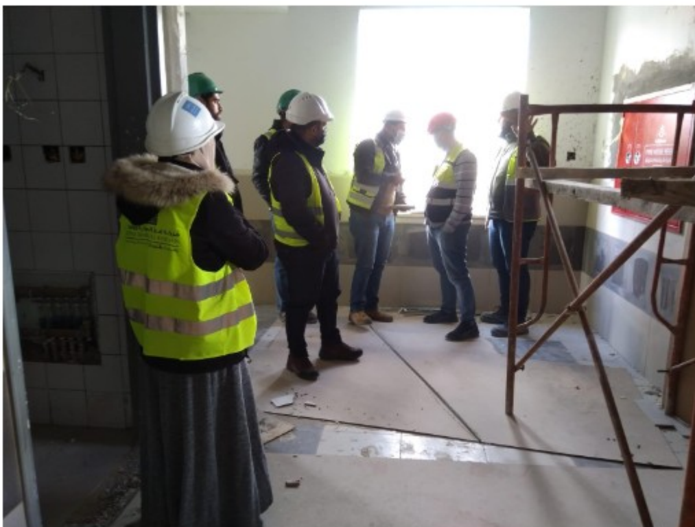
Eng. Odai preserving the fence from the window, commenting that some parts of the fence are clearly damaged and need fixing
