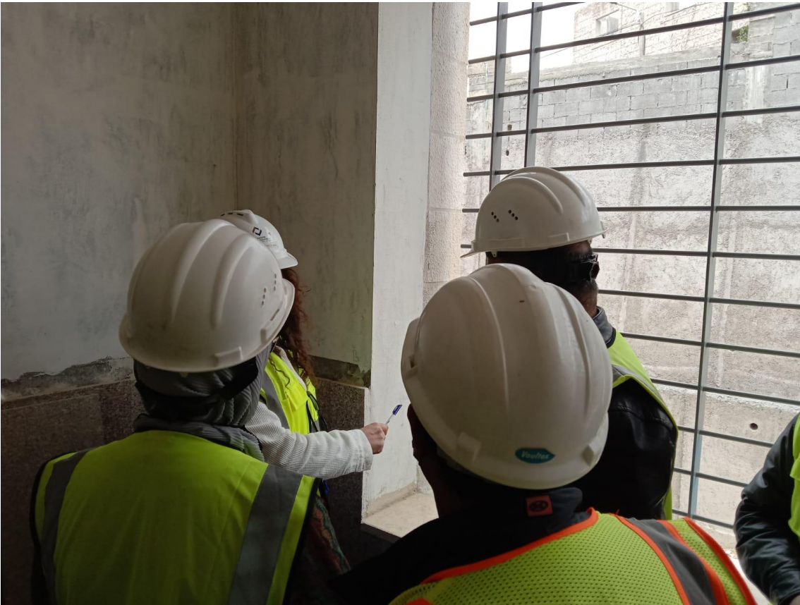
The team discussed with the Contractor the continuation of granite to the window jambs up to the aluminum frame
