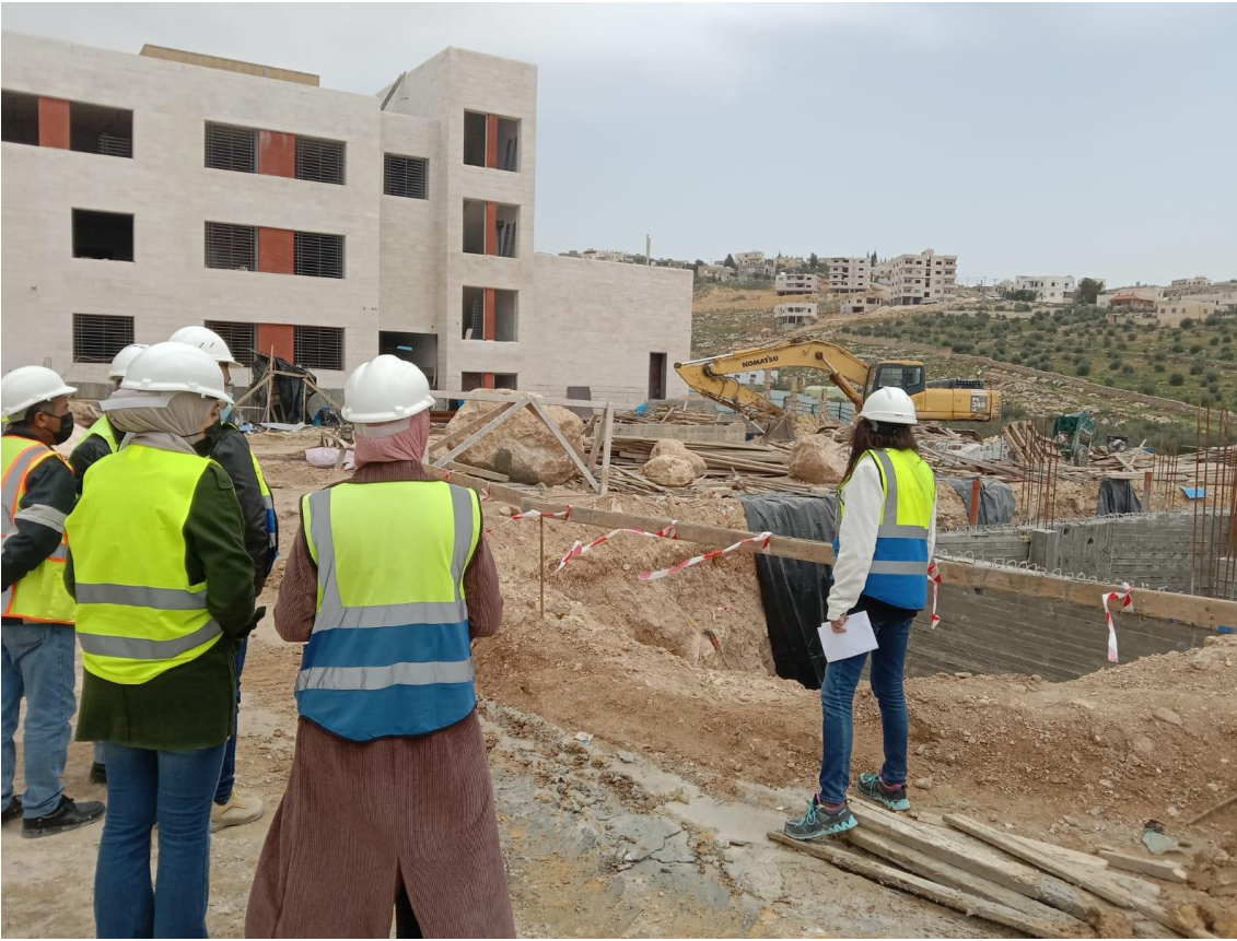
Inspecting the structural work ongoing for the guard room and main gate
