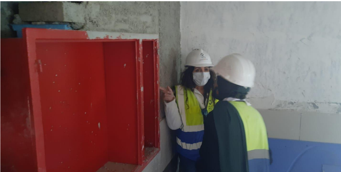
The Supervision team observed defects in the installation of the fire hose cabinets:
