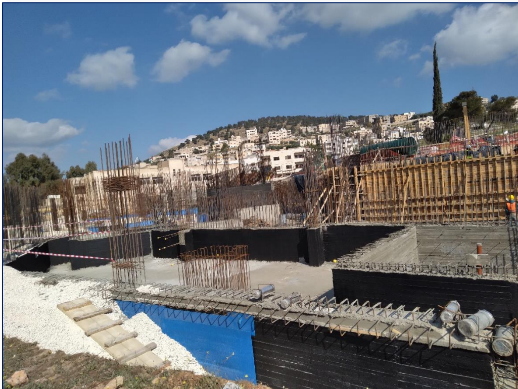
FIGURE #09& 10: Backfilling works is ongoing. Insulation works is ongoing. Photos credit: Talid Hamdan March 28 th , 2021
