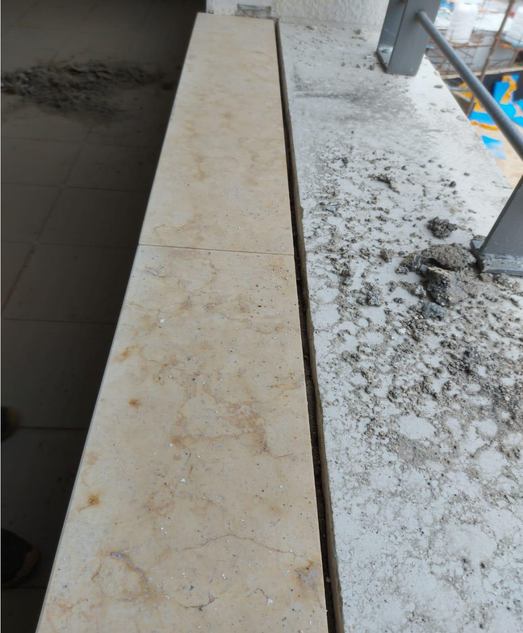
The gap between the two sills
