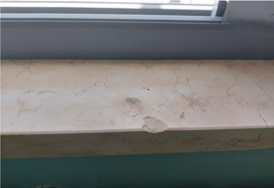
Broken edges of the window sills
