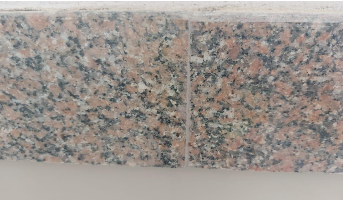
Replacing the unacceptable red grout for granite coping with the approved grout
