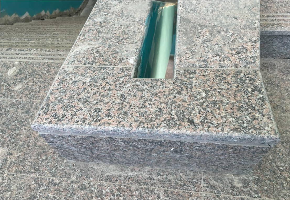
Replacing the small pieces of granite parapet cover of the staircase by larger suitable pieces
