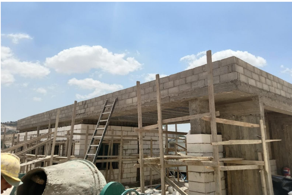
No stiffener columns in the parapet
