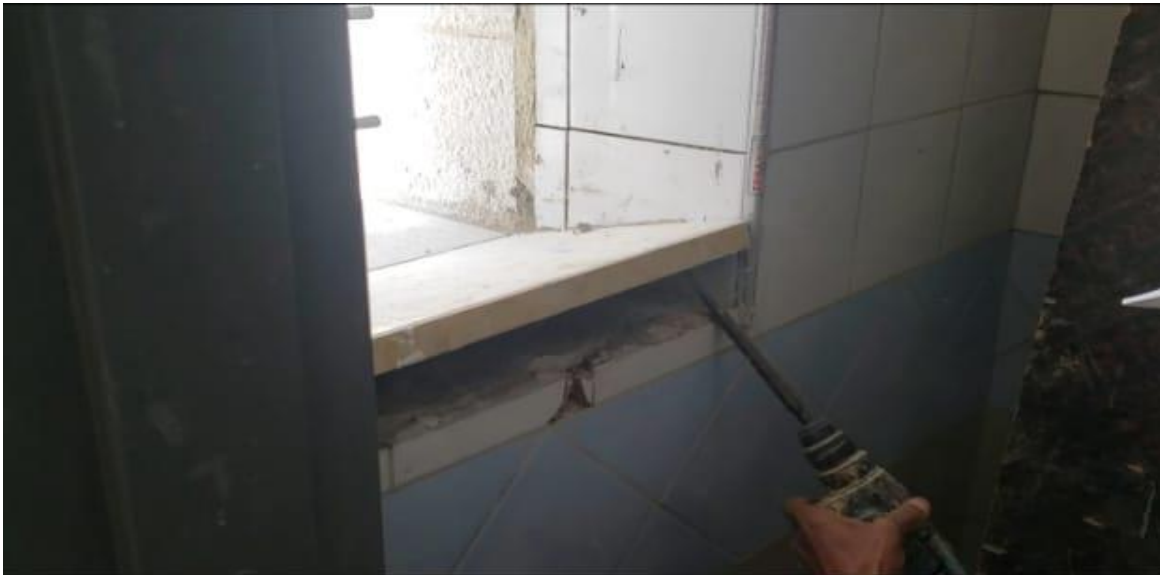
Removal of defected window sill
