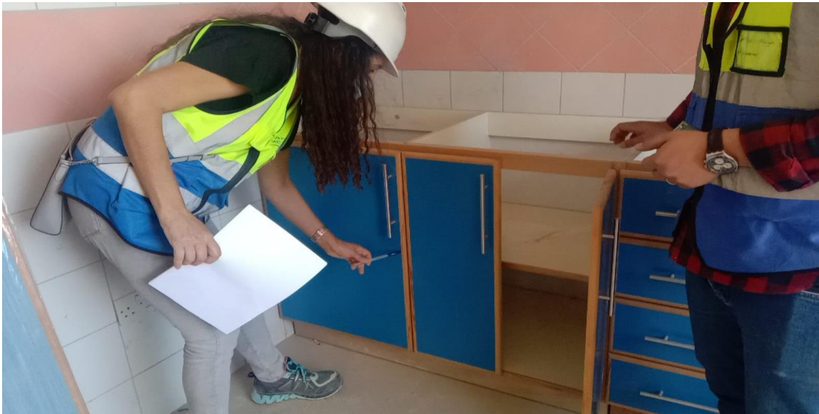
Defects in wooden cabinets
