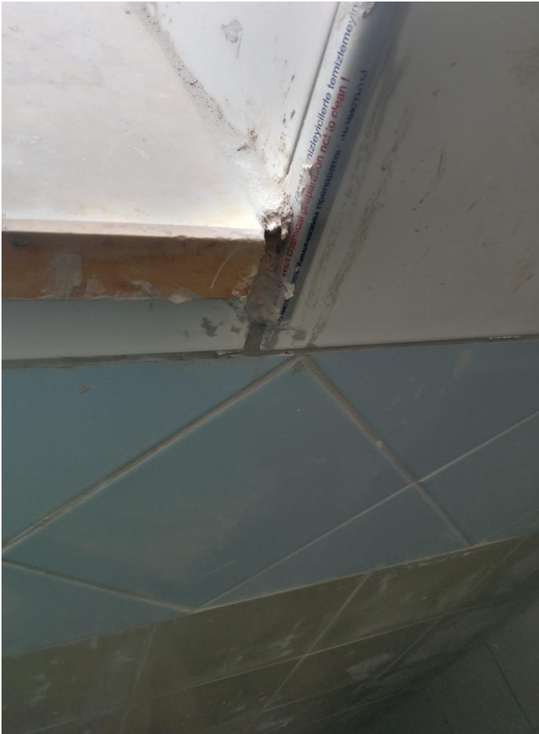
Wrong dimension for window sill
