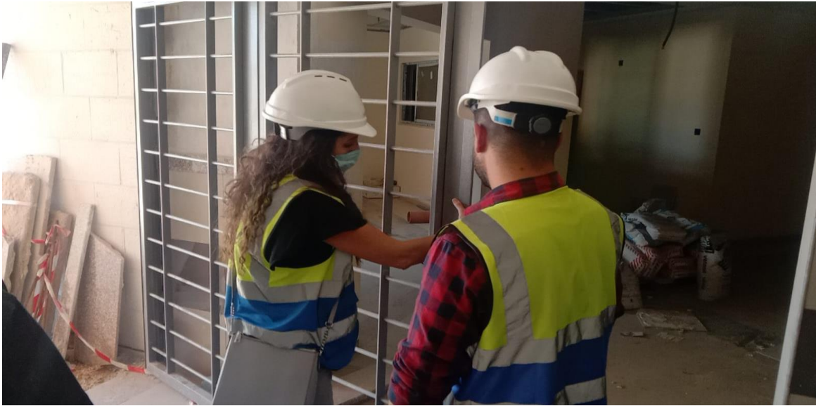
Defects in the main steel doors
