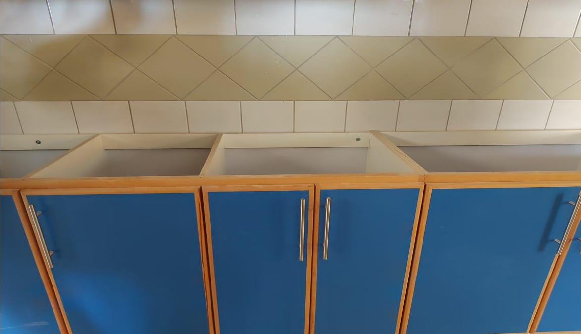
Defects in the beech frame and partitions
