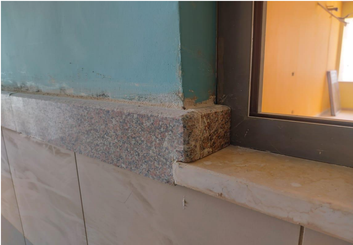
Defects in the granite coping
