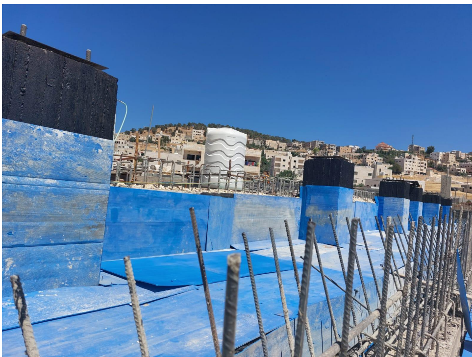
Installing carton boards for the foundation of the amphitheatre and columns of the shadings
