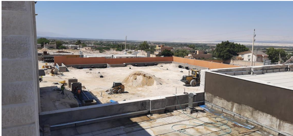
Insulation work at the roof of zone C and External works at the front area
