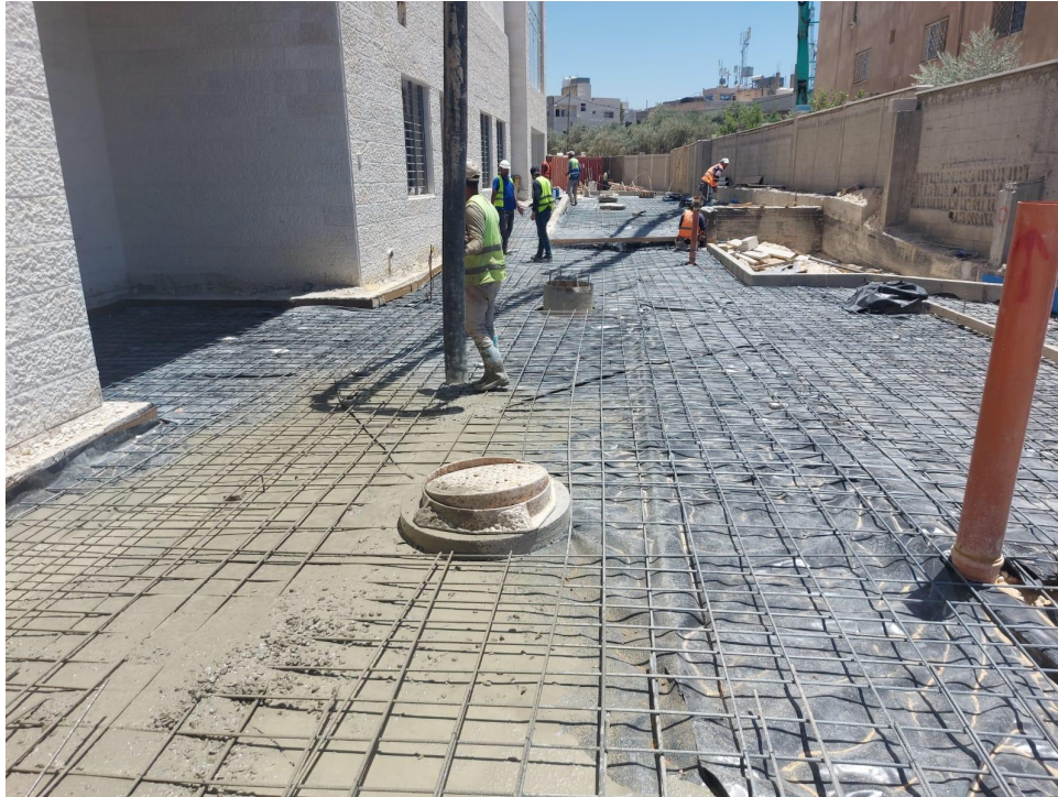
Casting concrete for the slab on grade at the southern side of the building
